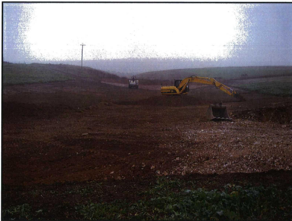
Plate 2: The subsoil strip, chalk bedrock exposed and reduced in foreground, view south-west
