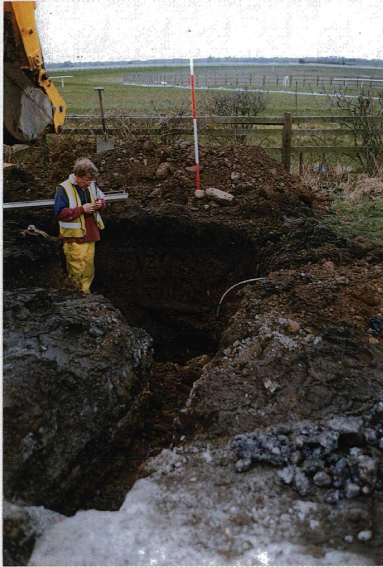
PLATE 2 TRENCH 3 WITH SOAKAWAY, SHOWING WATER MAIN IN SIDE OF TRENCH AND FORMER TARMAC ROAD
