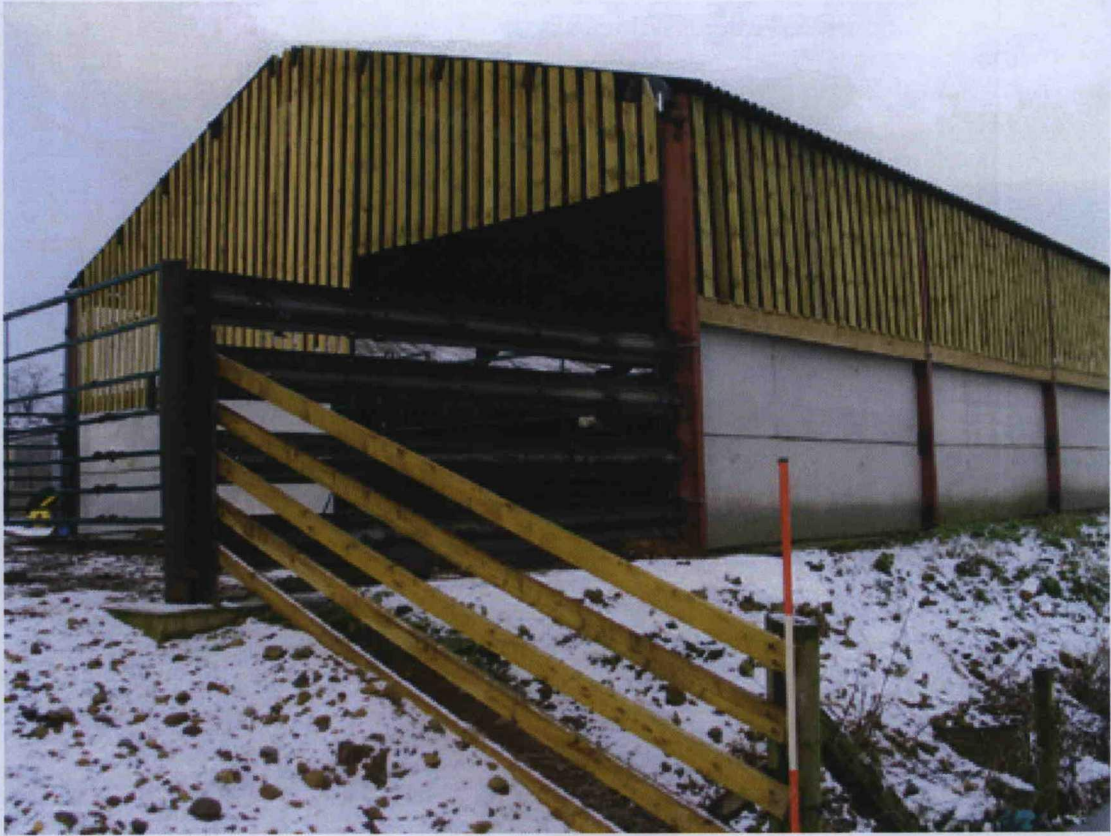
Pl. 2 To show the stone foundation upon which the barn was built, looking NW
