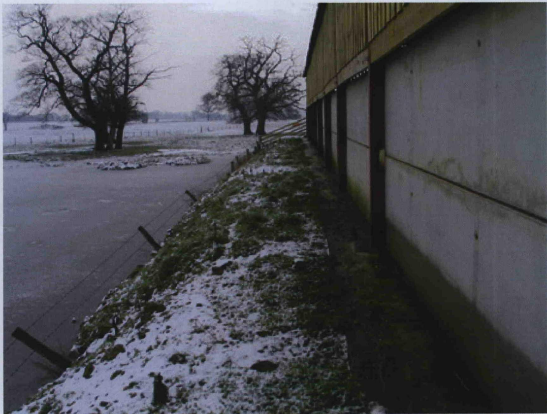
Pl.3 To show the barn upon a stone foundation, looking SE towards the moat
