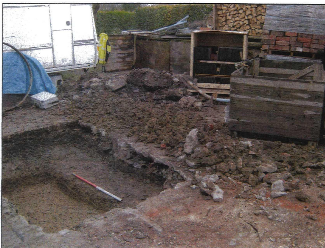
Plate 1. General View of Evaluation Area, looking south-west. Trench 1 in foreground, Trench 2 to right of hi-viz jacket.
