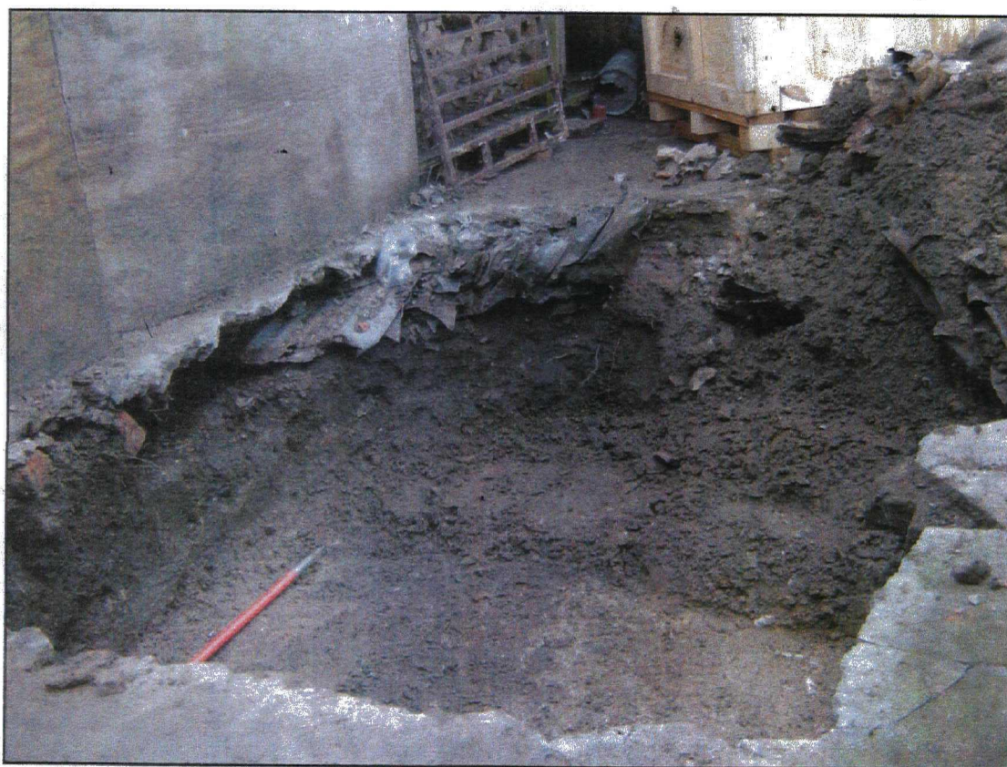
Plate 6. Trench 2, showing problems with dumped material and access. Looking east, scale 1m.
