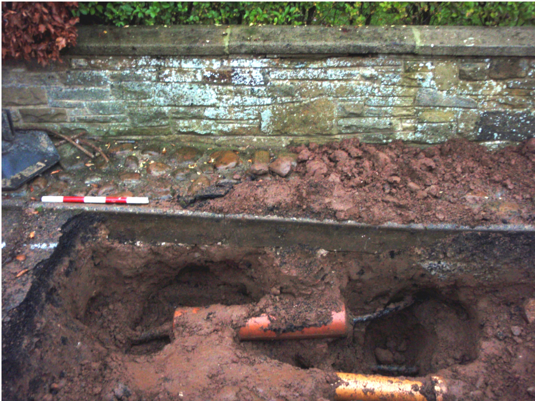
Plate 11 View of maze of services in part of NE pavement trench, looking WNW
