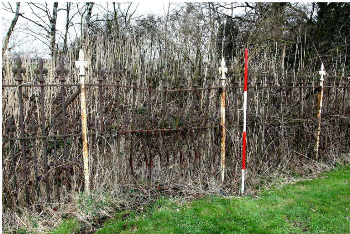
Plate 14 Damage to E – W stretch of park railings, looking NNE
