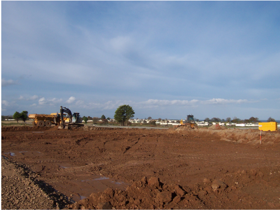
Plate 5 The reduction of the ridge in the vicinity of the contractor's car park, looking north-east
