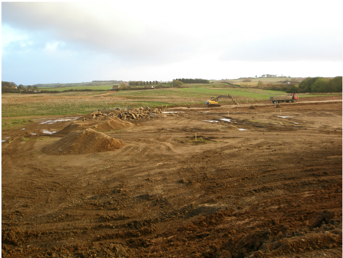
Plate 4 General shot of stripping and ground reduction in the western part of the site, looking south
