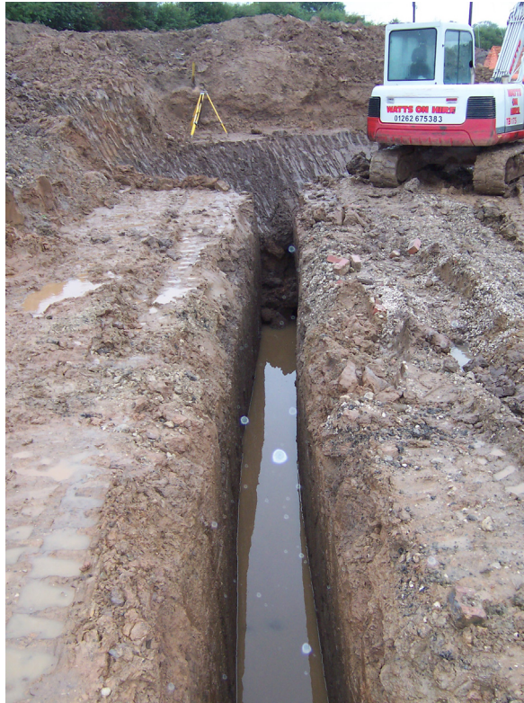
Plate 3 The culvert trench to the north of the open drainage channel, looking south
