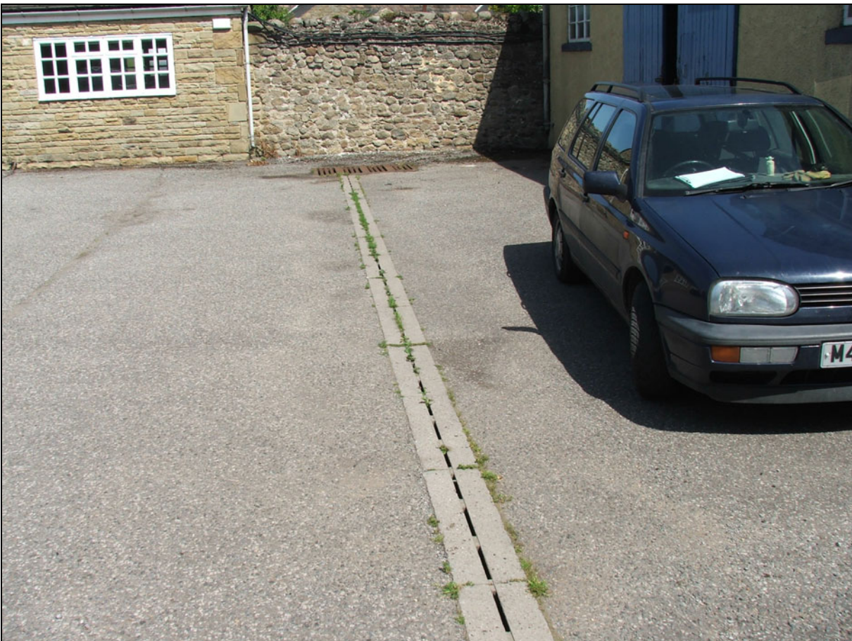
Plate 4. Services and drainage in the forecourt
