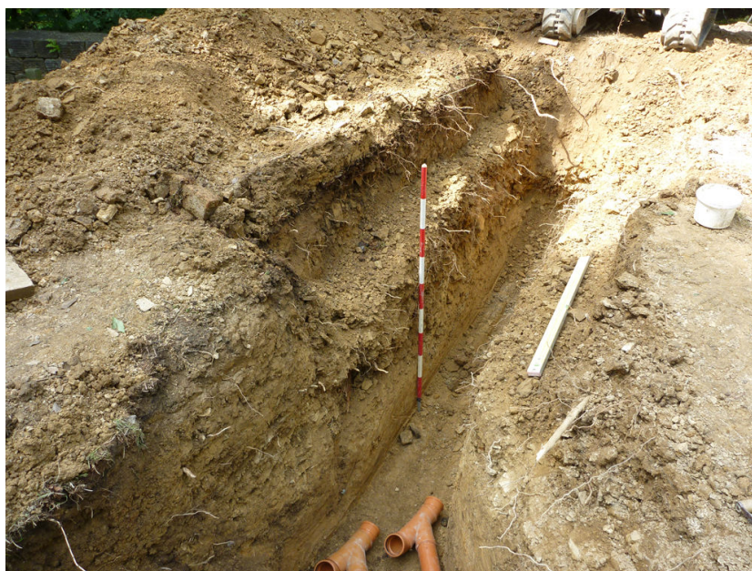
Plate 10 Western part of service trench, showing widening and stepping, and the limit of the graveyard soil beyond the photographic scale
