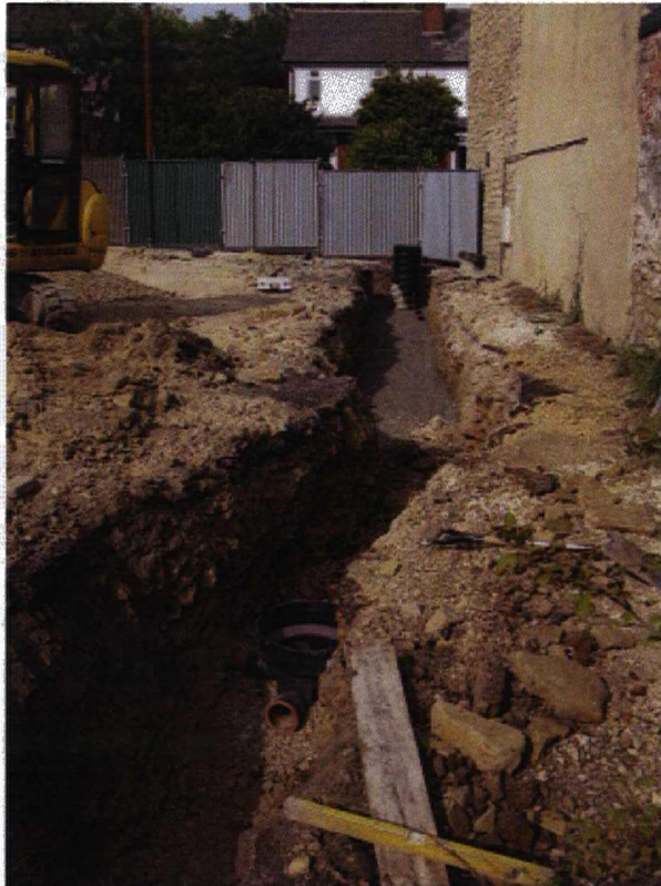
Plate 5 The foul drainage trench connection, part-way through excavation. Viewed from the south.
