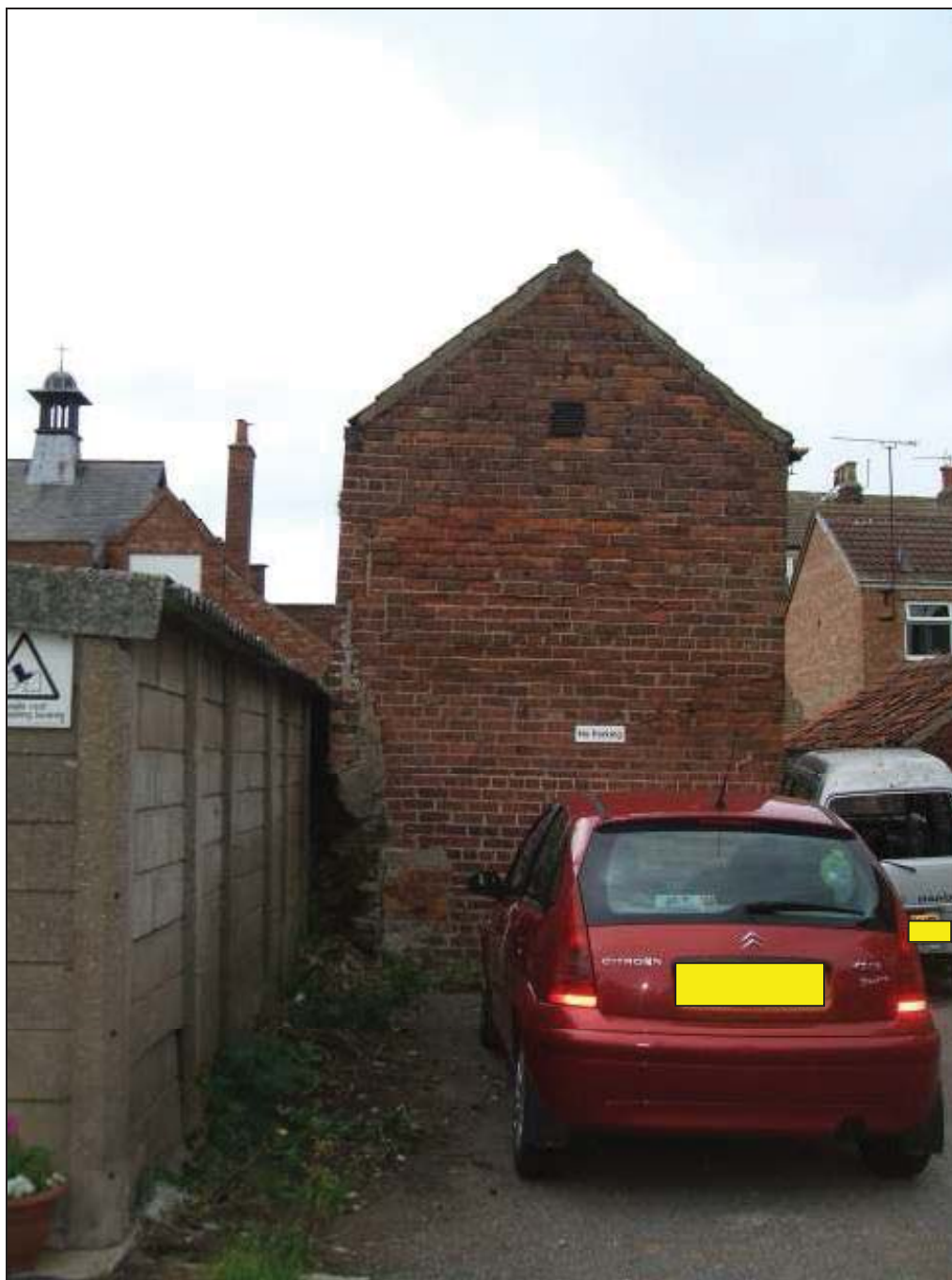
Plate 7 Brick structure towards north-east corner of site, possibly associated with fish curing, looking north-north-east
