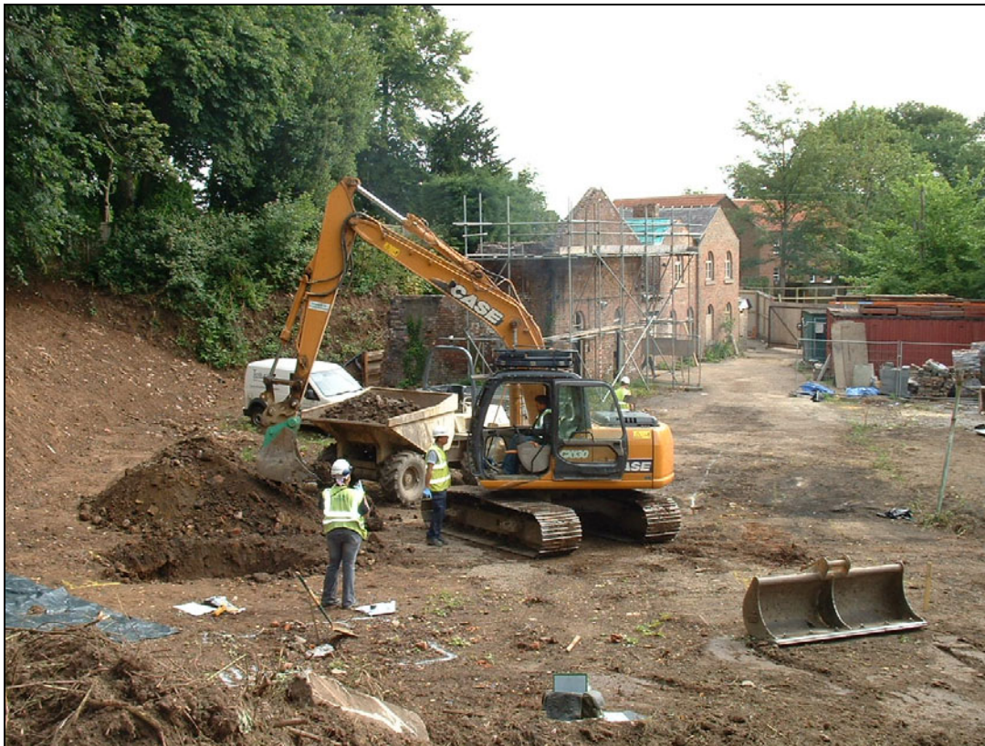
Plate 1. General site shot looking north
