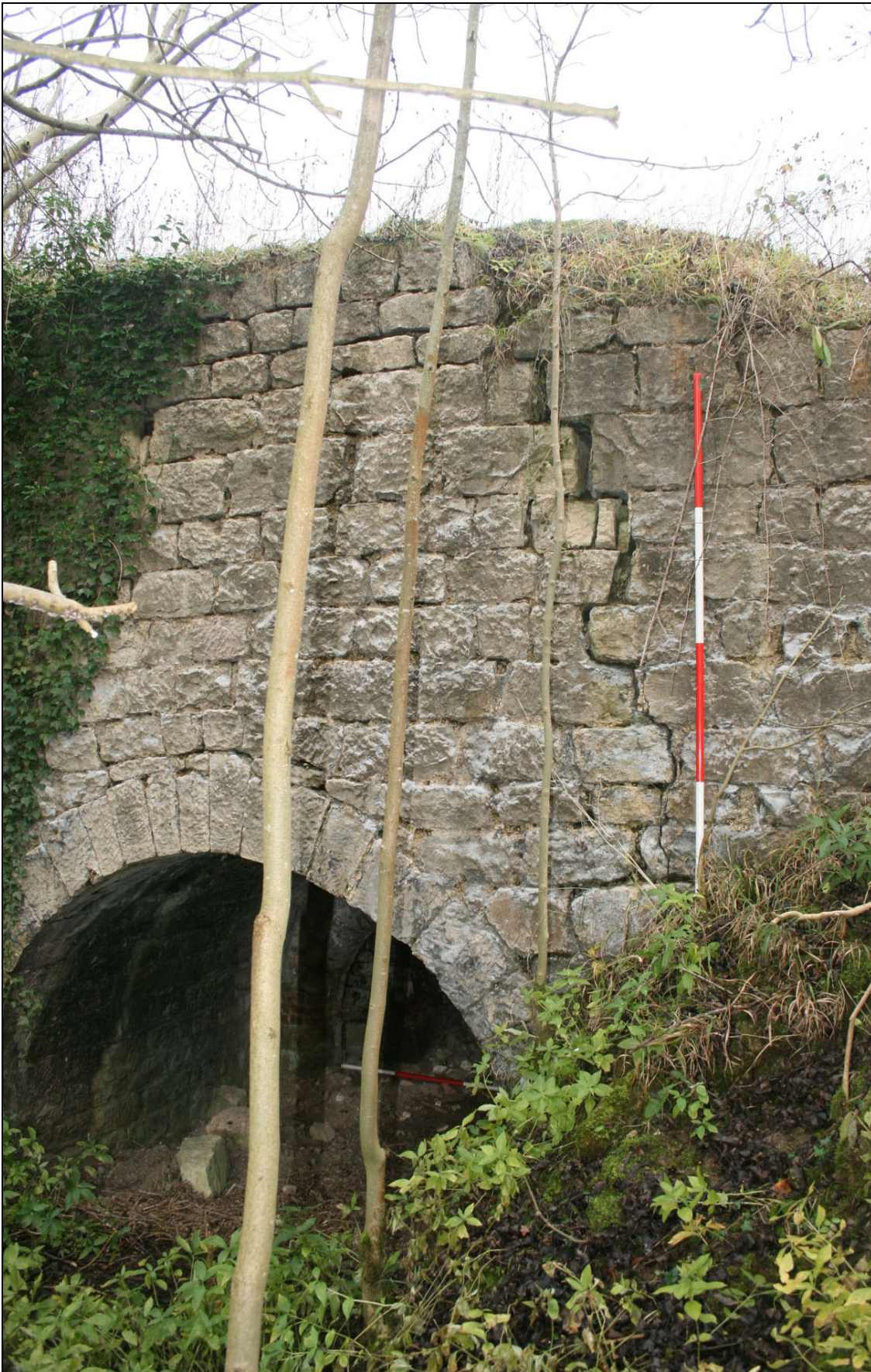
Plate 11. The crack in the facade of Kiln C
