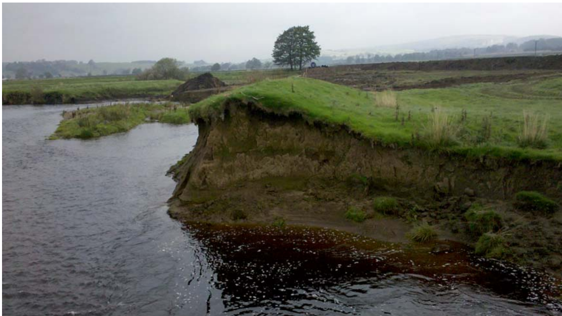
Plate 2: The result of severe riverine erosion, which has truncated a portion of embankment 101=105 , looking north
