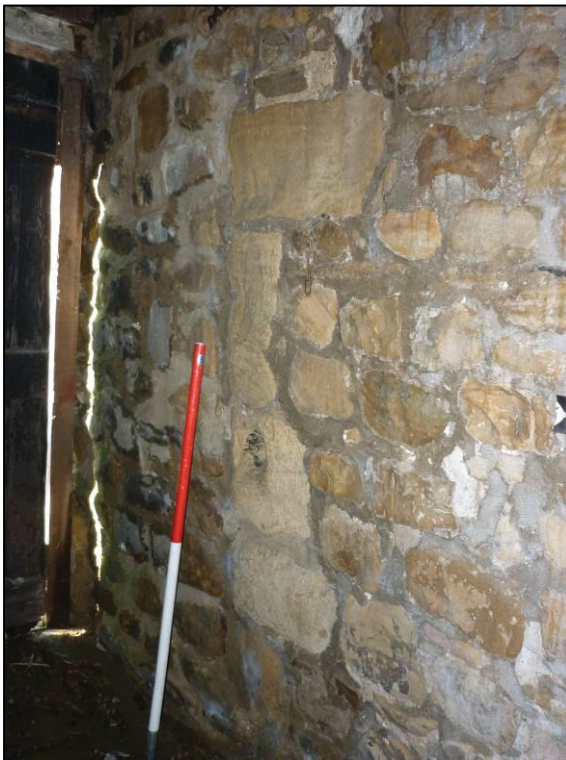
Plate 2: Medieval building, blocked doorway in base of south gable, looking NW (photo 3/827).
