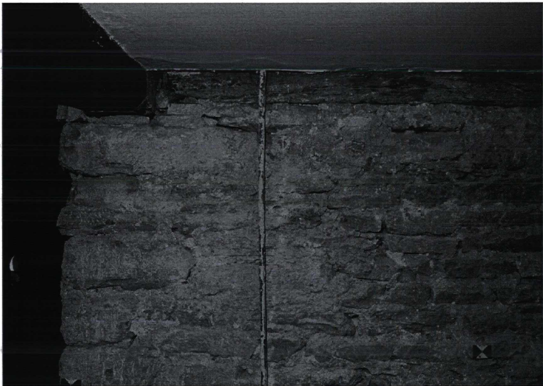
Plate 4 West Face of Passageway Wall – ceiling timbers at the north end of the wall
