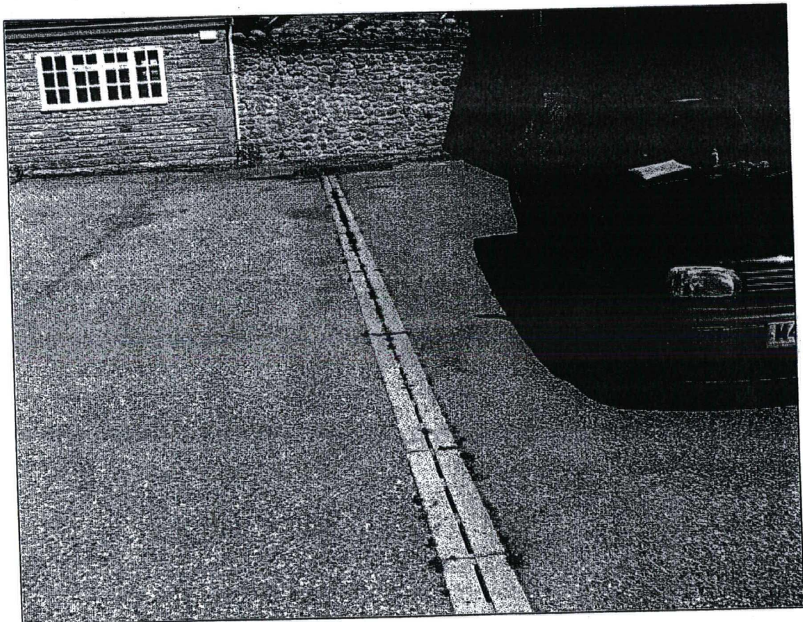
Plate 4. Services and drainage in the forecourt
