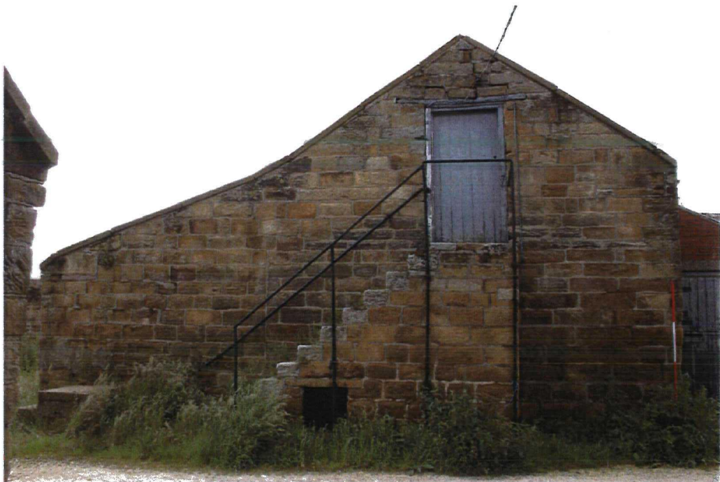
Plate 8 Building 14, E elevation. Steps to loft with kennel and store under. Stable extension to left (note mounting block) and later brick extension to right. Looking W
