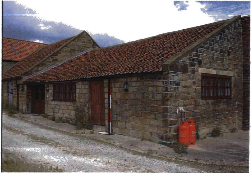
Plate 15 Building 20, W elevation to left, S elevation to right. Converted to holiday accommodation and ribbon-pointed with hard cement. Looking NNE
