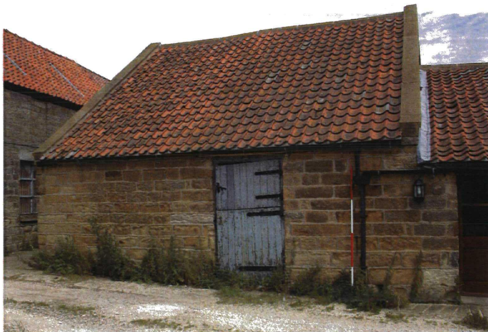
Plate 14 Building 19, W elevation, Building 15(A) to left and Building 20 to right. Note continuity of stone coursing between 19 – 20. Looking NE
