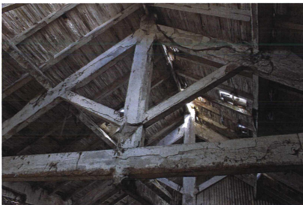
Plate 4 Building 10, detail of king-post roof trusses; roof covering of pantile over laths secured to rafters.
