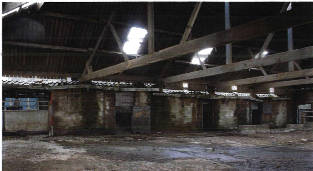
Plate 1 Part of S elevation of Building 6, roofed fold-yard of Building 9 over. Looking N
