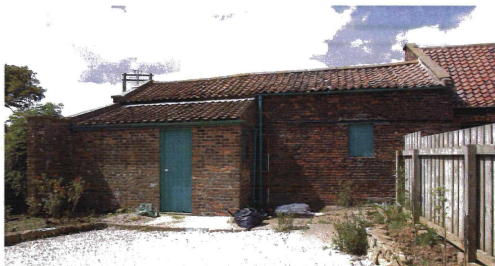
Plate 18 Building 21, E elevation, extension 21C to left foreground, 21B behind and 21C to right. Looking W
