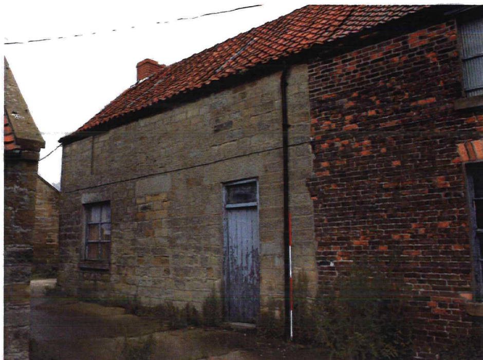
Plate 11 Building 15 (A). The stone S elevation of dwelling with 2 blocked openings to first floor and 1 to ground floor. Note dwelling extended into barn to right. Looking W
