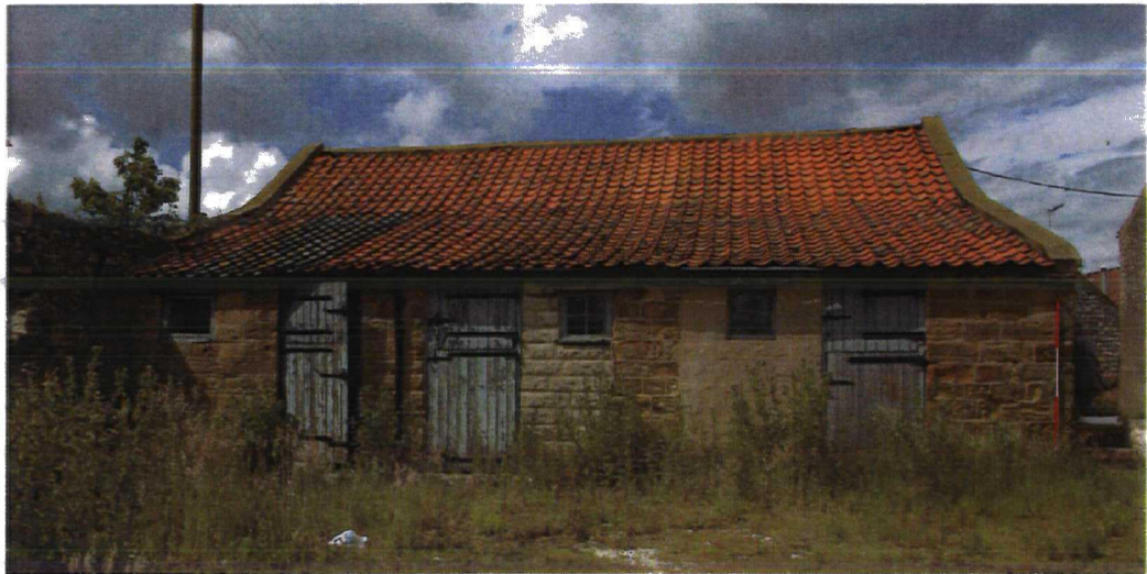
Plate 9 Building 14, S. elevation (stable block extension) note change in roof pitch. Looking NNW
