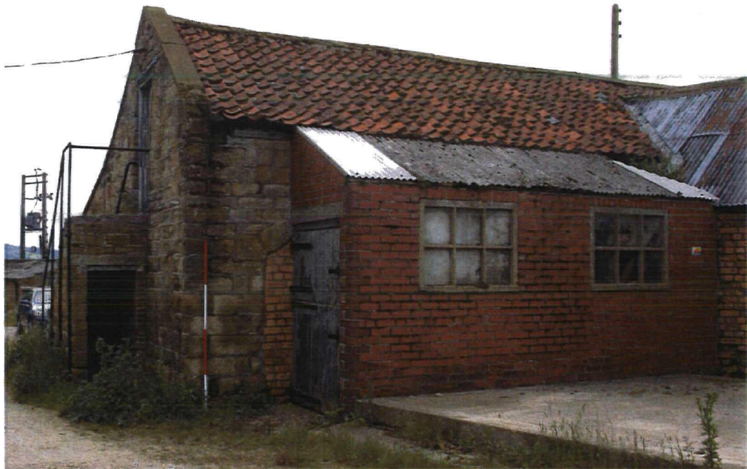
Plate 10 Building 14, N elevation. Showing 30 th century brick extension with concrete windows. Note that this extension masks much of the blocked-up eastern arcade of the old core of Building 14. Looking S
