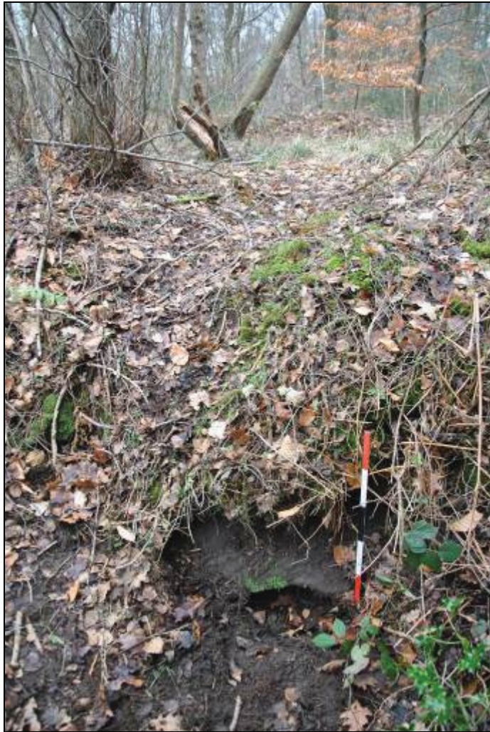
Figure 22 (left) The lintel of a culvert on the upstream side of the west dam. This links with the stone-lined shaft, which is marked by the vertical logs at top centre of the picture
