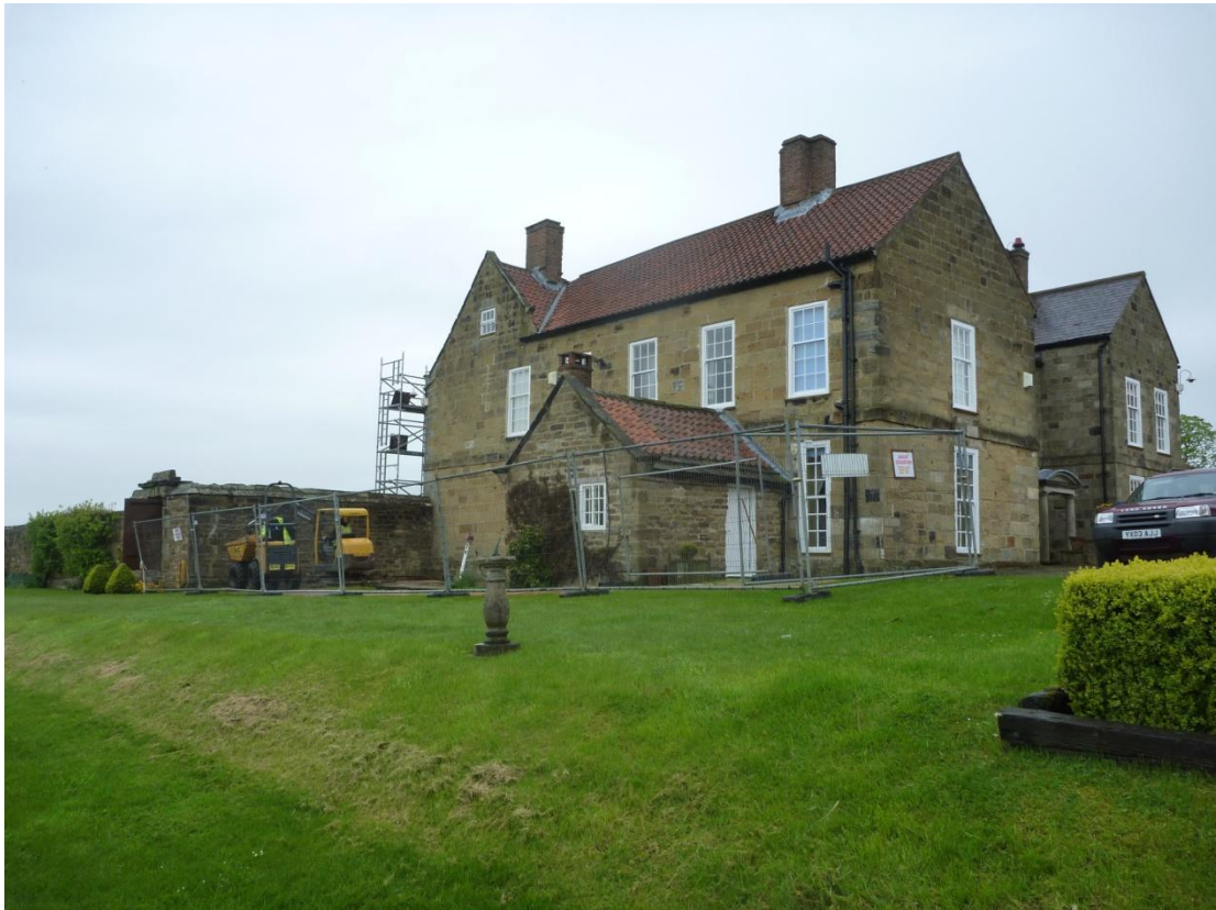
Plate 1 View of house and works for library extension. Note terracing in foreground. Looking NW.
