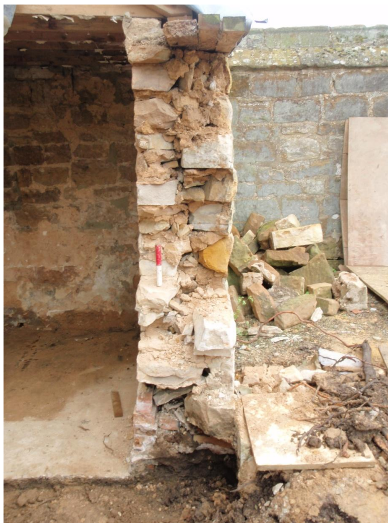
Plate 8 Cross section of store walling after removal of the east wall. Looking W.
