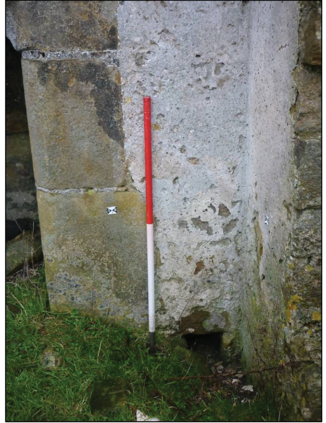
Plate 15: Plaster and drain to east of fireplace FP1 in elevation 16, looking N (photo 2/556).
