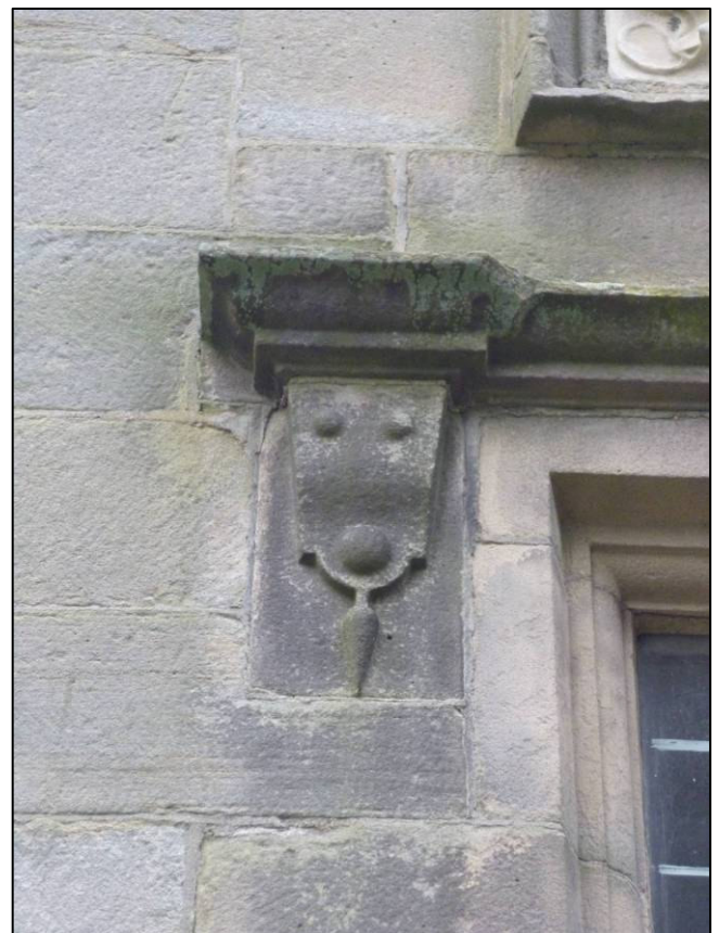
Plate 27: Weston Hall Banqueting House, first floor window detail on west elevation, looking E.
