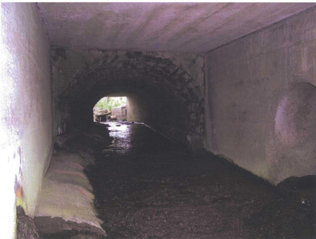
Plate 32: SCA2: beneath Cloven Hill bridge/culvert, showing the earlier stone-built arch, perhaps part of an earlier bridge, incorporated into the later structure
