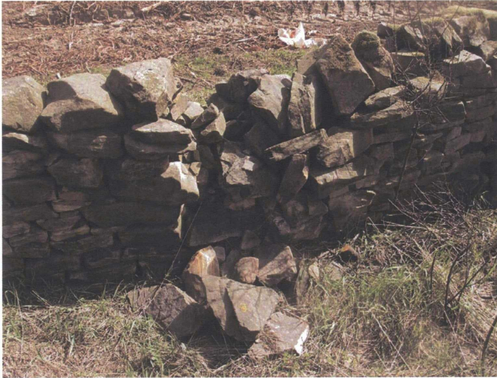
Plate 80: Site 017, showing details of wall collapse at the lay-by on Stephen Bank
