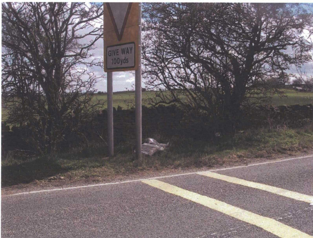
Plate 77: Site 014, wall on Lanehead Lane, to the north of the carriageway, looking south. The wall is in very degraded state
