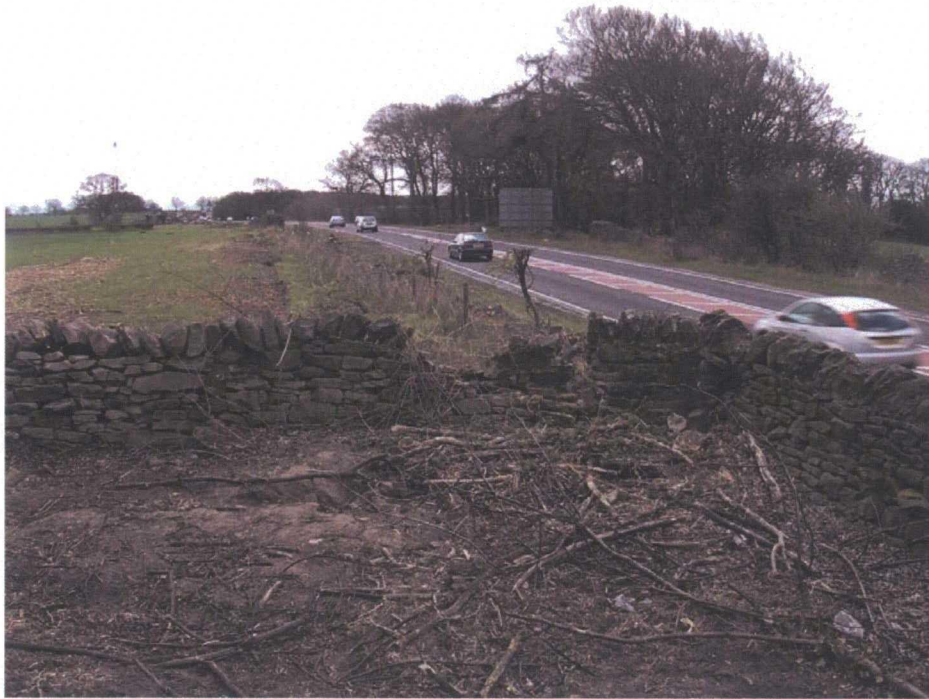
Plate 64: Site 001, the eastern end of Gatherley Moor Quarry, from the north of the carriageway, looking south-east. Wall in state of disrepair, large sections missing
