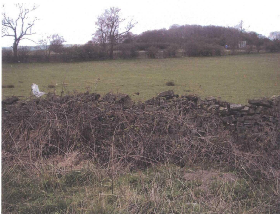
Plate 73: Site 010, field wall to the south of the carriageway taken on Forcett Lane, looking south. As with 009, it appears to have been poorly rebuilt and shows signs of deterioration. Note the lack in quality of its construction compared to examples at Gatherley Moor Quarry
