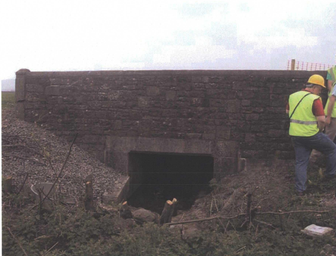
Plate 84: Site 021, stone headwall for a culvert at the south of the carriageway to the south-east of Carkin Moor Roman fort. The structure is roughly 2.5m in height, and is likely to be of late twentieth-century construction
