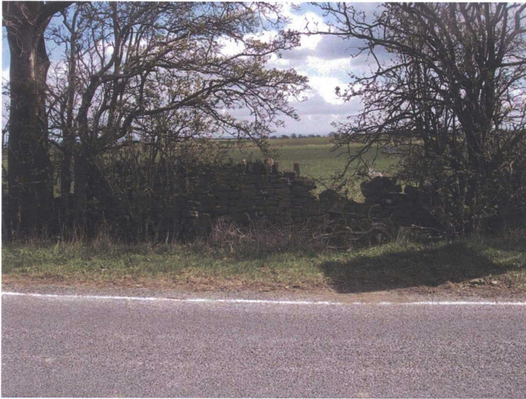
Plate 76: Site 013, field wall at Stephen Bank, to the north of the carriageway on New Road, looking south-west. Similar construction to walls at 011 and 012, but in a very poor state of repair
