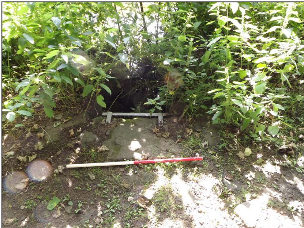
Figure 15. Outflow at southern end of dam, scale 1m
