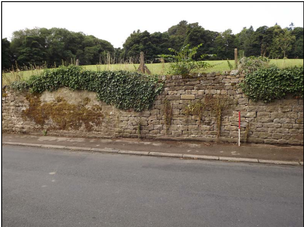
Figure 10. Possible rebuilt gateway for path to ice house (Site 5), scale 1m, looking NW
