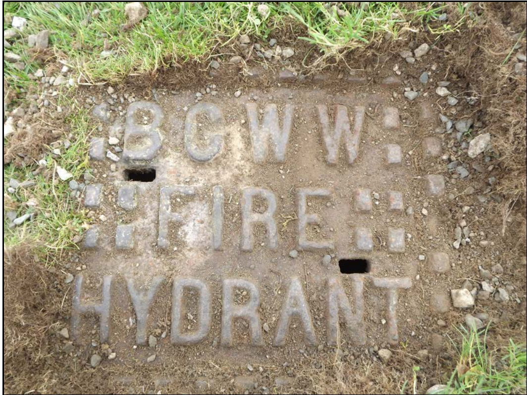
Figure 18. Part of fire hydrant supply system
