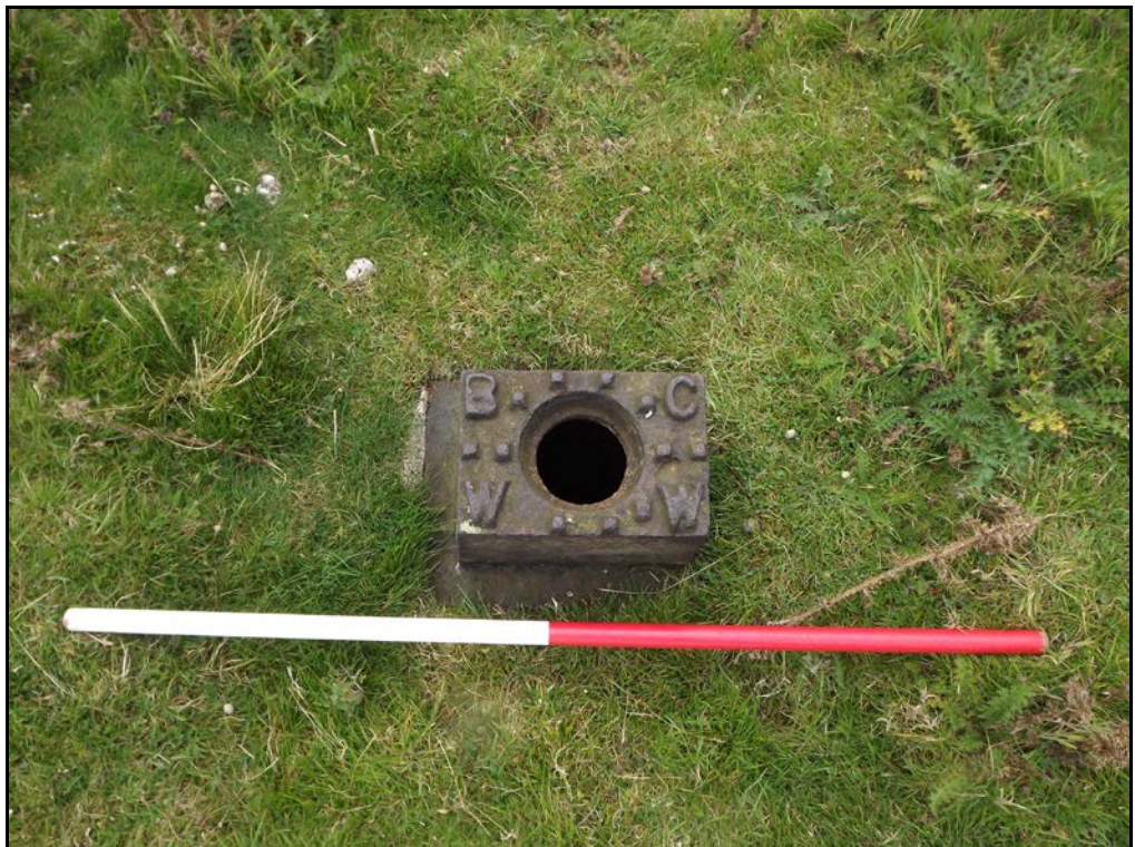
Figure 17. Part of water supply system, scale 1m
