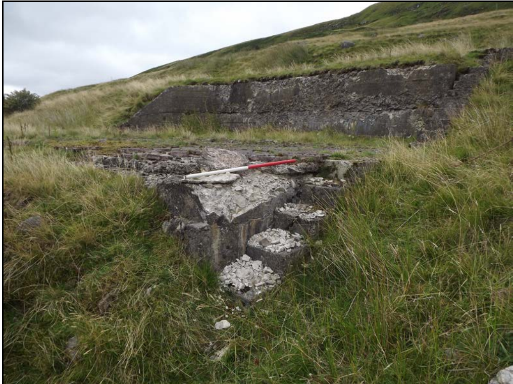
Figure 19. Recent loss of structure in one of the hostels, scale 1m, looking SE
