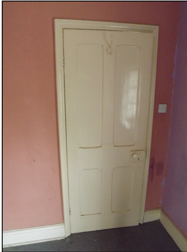
Plate 8. Door in main bedroom with original lock and coat hook, looking south-west
