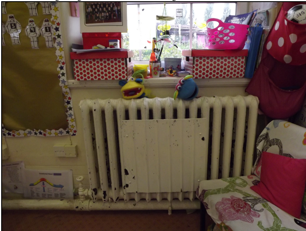
Plate 30. Original cast iron radiator, looking south
