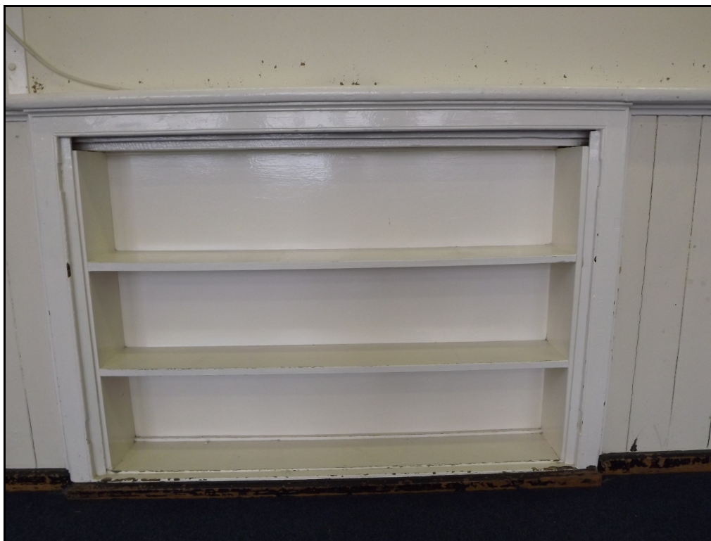
Plate 26. Detail of an original built in wooden cupboard in one of the classrooms
