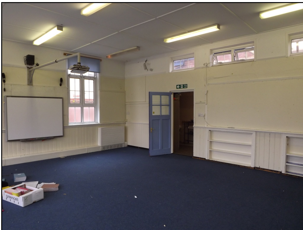
Plate 25. Interior of classroom on eastern side of block, showing surviving wooden panelling, door and remains of built in cupboards
