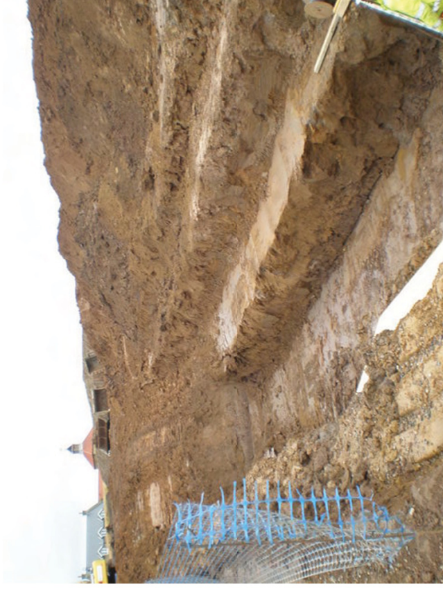
Plate 2. Section through Pipe Line Excavation Trench (Northern end of WwTW). Facing North-east.
