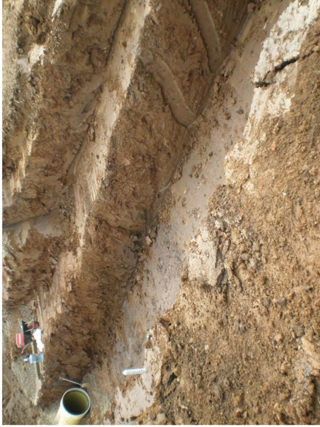
Plate 3. Section through Pipe Line Excavation Trench (Central Area of WwTW). Facing North-west.
