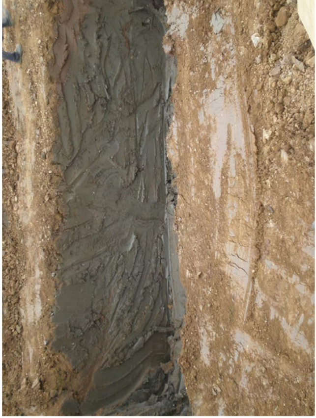
Plate 5. Section through Pine Line Excavation Trench. (Southern end of WwTW). Facing North.
