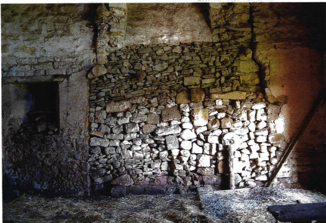
Plate 8. Northern Firehood. Facing North.
