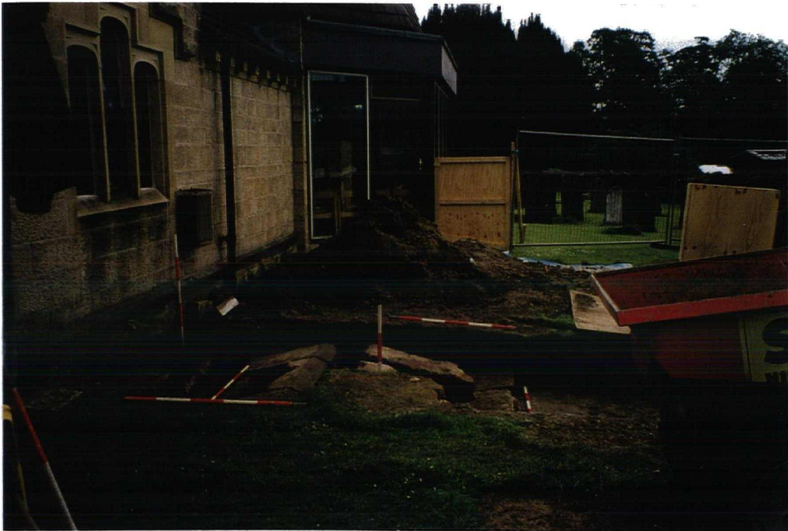
Initial phase of groundworks, exposing relocated sarcophagus plinth and foundations of in-situ funerary monument.
