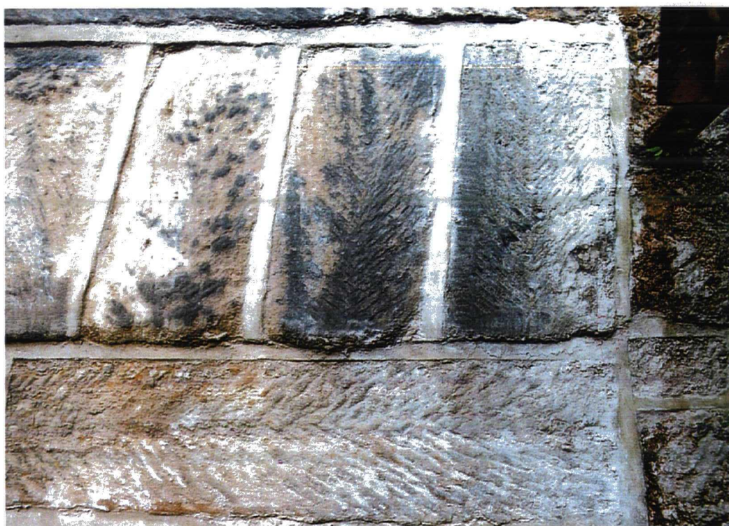
Plate 15. Old Sail Loft – Sail Loft range, detail of herringbone masonry with margined block visible to right
