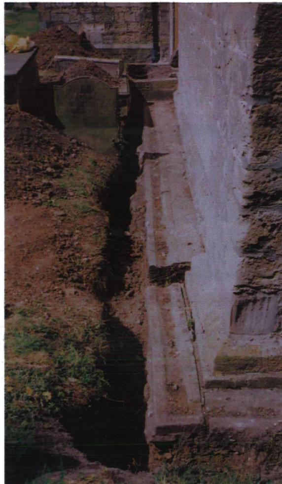
Plate 2 New drainage trench and contexts 1000 and 1001 adjacent to the south side of the chancel
