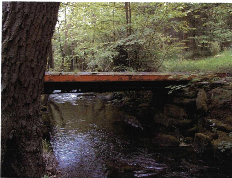
Plate 5, Up-stream side of the Iron footbridge across the river Skell, supported on stone piers constructed on the north and south banks.
