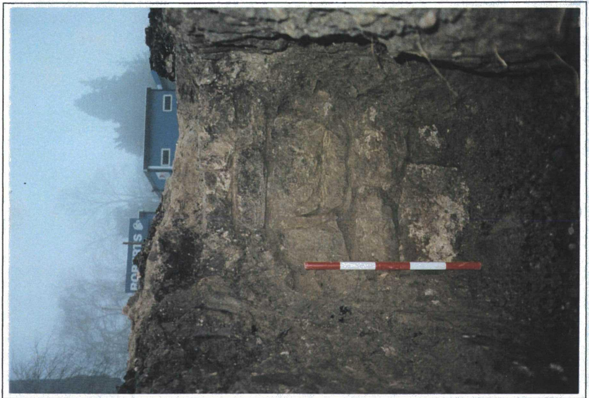
Plate 3. North-facing elevation of wall [52] prior to dismantling for drainage trench. Scale 0.50m.
