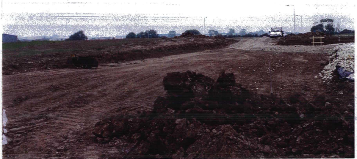
Plate 3. Site F. Area to the north of new build, proposed access road. Facing east.
