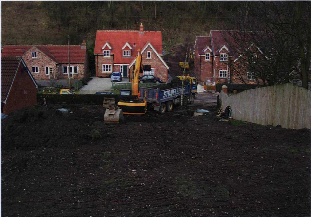
Plate 9. View of site during on site works, showing location of interceptor tanks. Facing north.
