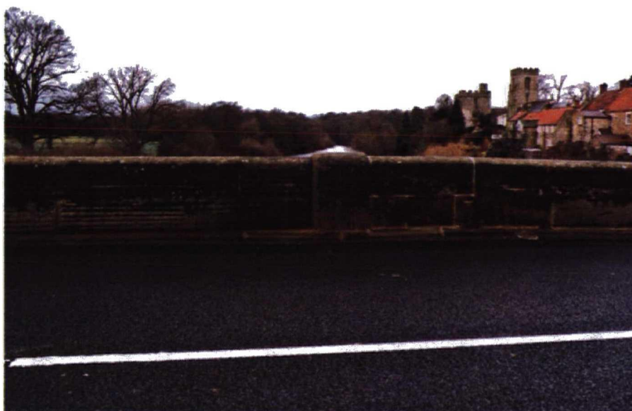
Plate 3: The inner, east side of Tanfield Bridge from showing the division between the North and West Ridings
