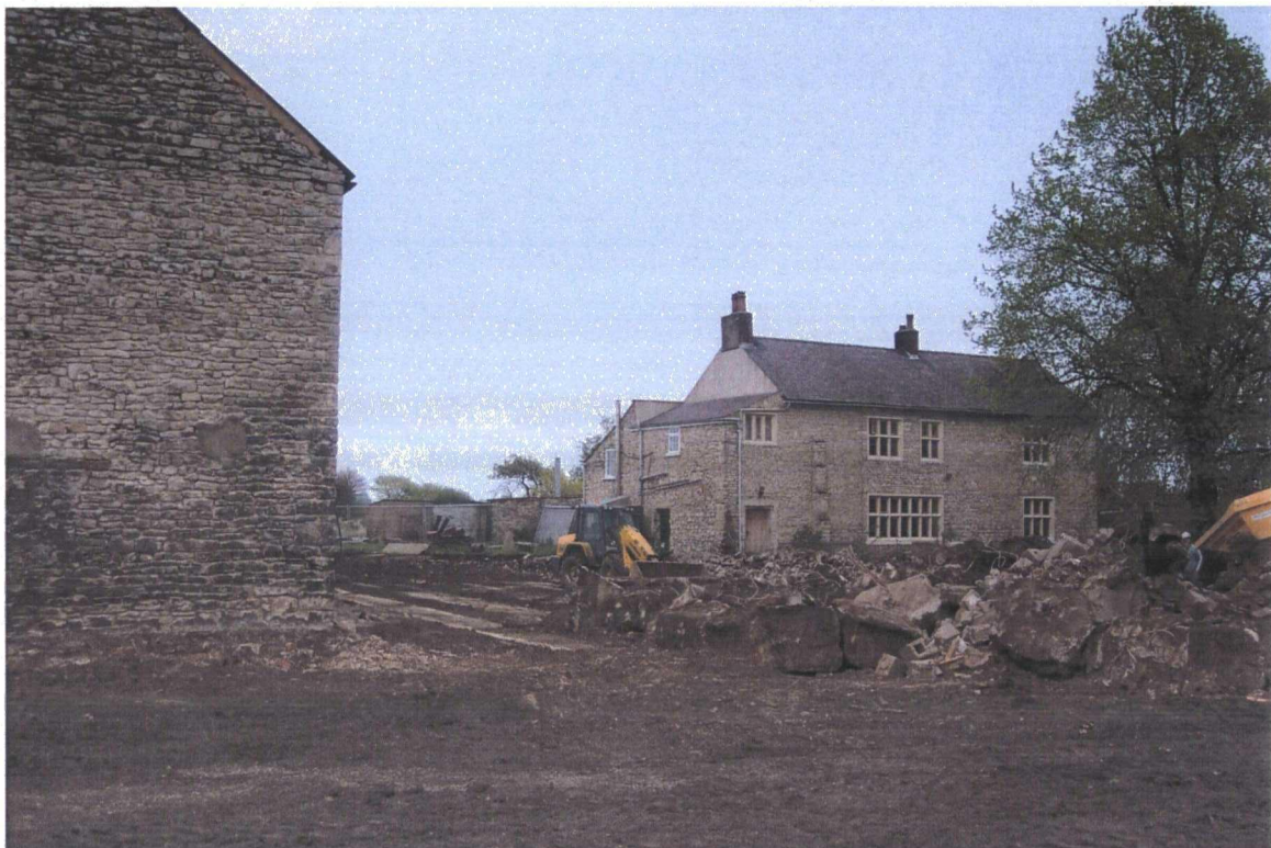
Plate 32. View to South of Barn after Demolition in this Area, Facing South West
