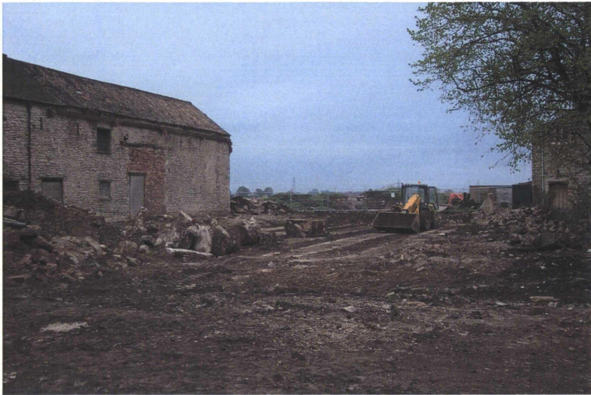
Plate 29. View to South of Barn after Demolition in this Area, Facing East
