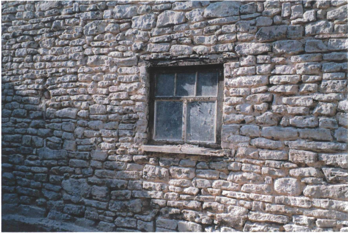
Plate 80. External View of Old Barn after Demolition of Brick and Corrugated Iron Structures
