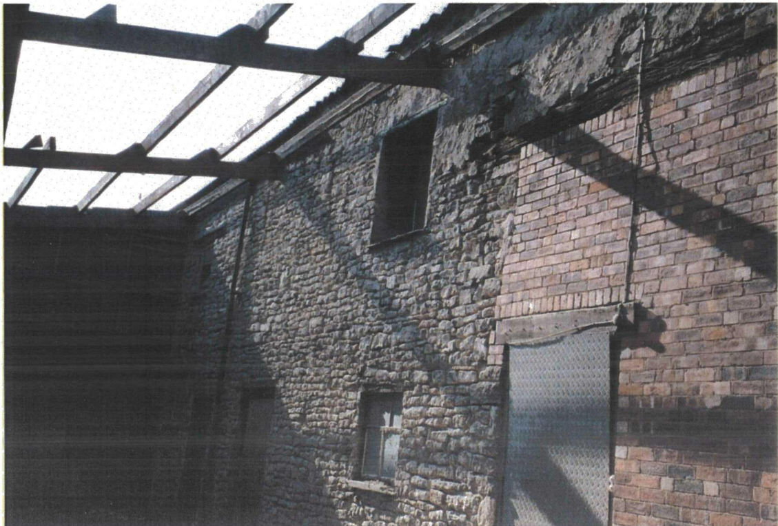
Plate 77. External View of Old Barn after Demolition of Brick and Corrugated Iron Structures
