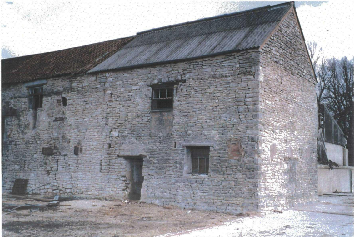
Plate 71. External View of Old Barn after Demolition of Brick and Corrugated Iron Structures
