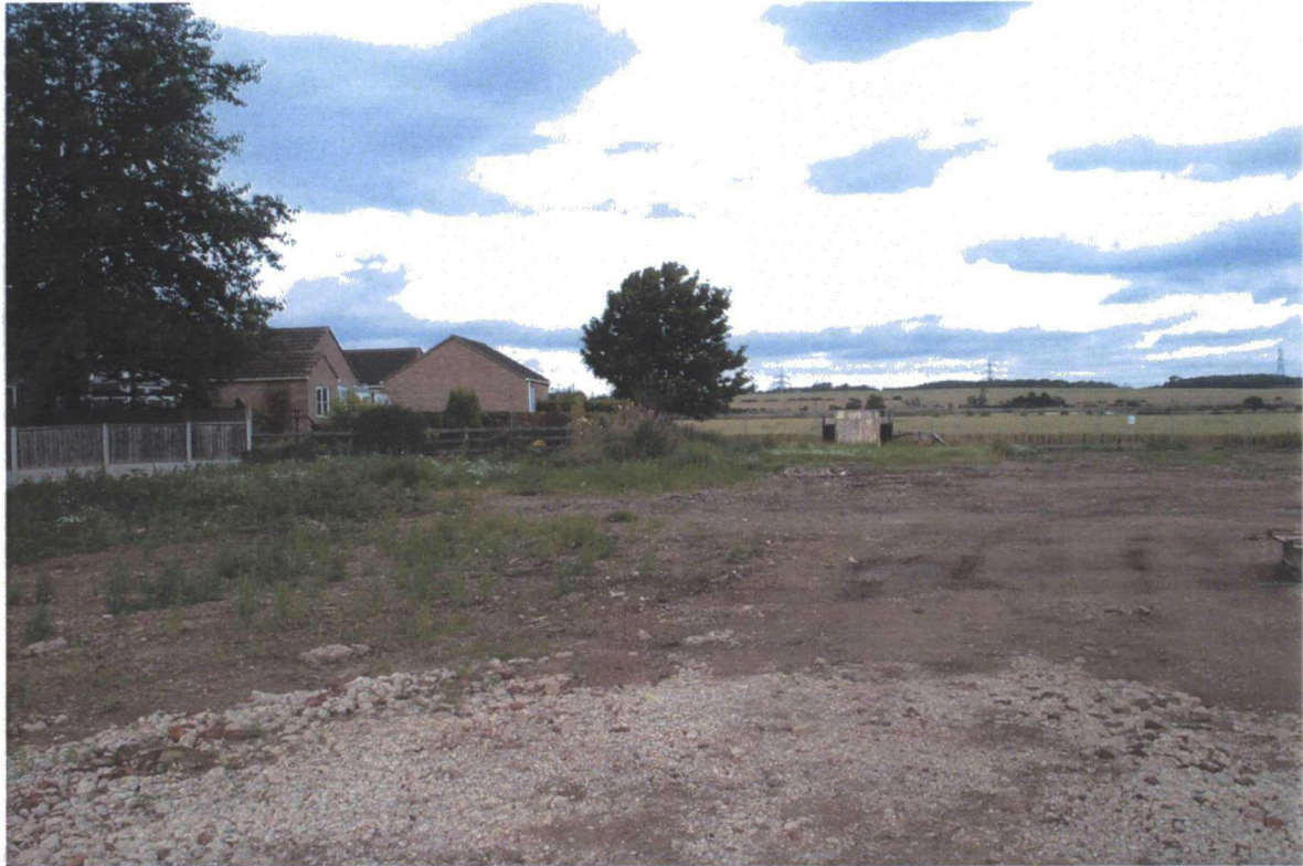
Plate 96. External View of Old Barn after Demolition of Brick and Corrugated Iron Structures
