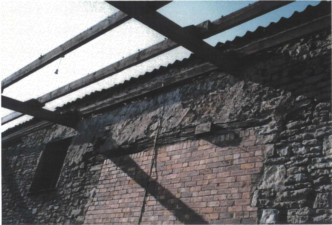
Plate 76. External View of Old Barn after Demolition of Brick and Corrugated Iron Structures
