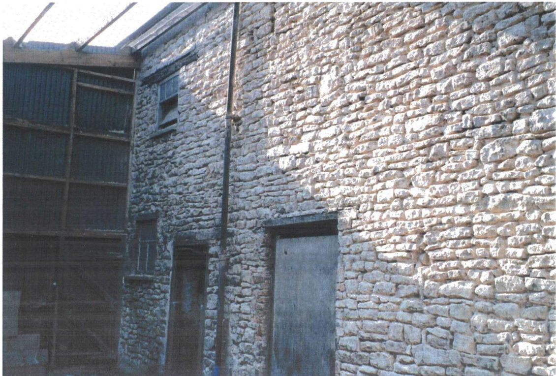
Plate 79. External View of Old Barn after Demolition of Brick and Corrugated Iron Structures
