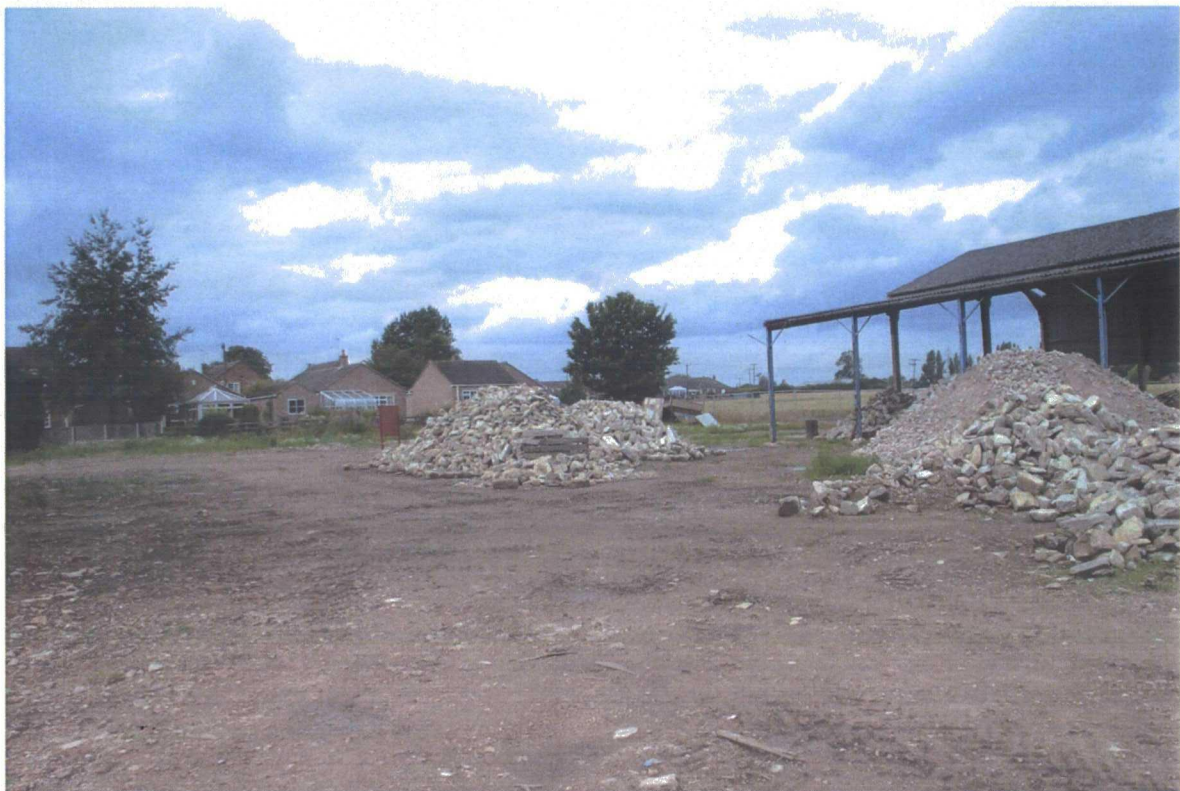
Plate 95. External View of Old Barn after Demolition of Brick and Corrugated Iron Structures
