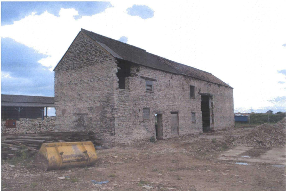
Plate 97. External View of Old Barn after Demolition of Brick and Corrugated Iron Structures
