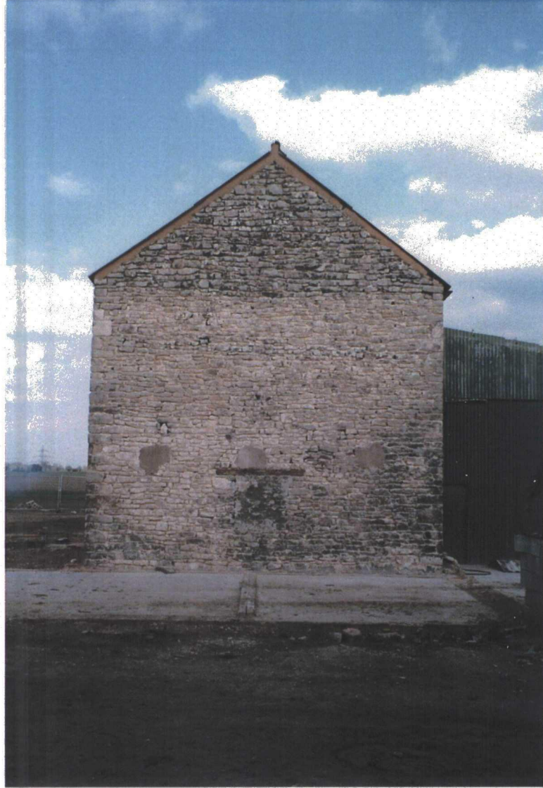
Plate 75. External View of Old Barn after Demolition of Brick and Corrugated Iron Structures
