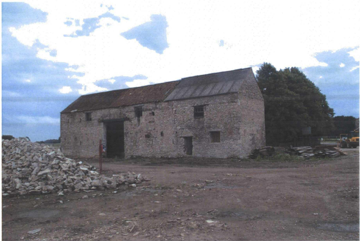
Plate 98. External View of Old Barn after Demolition of Brick and Corrugated Iron Structures
