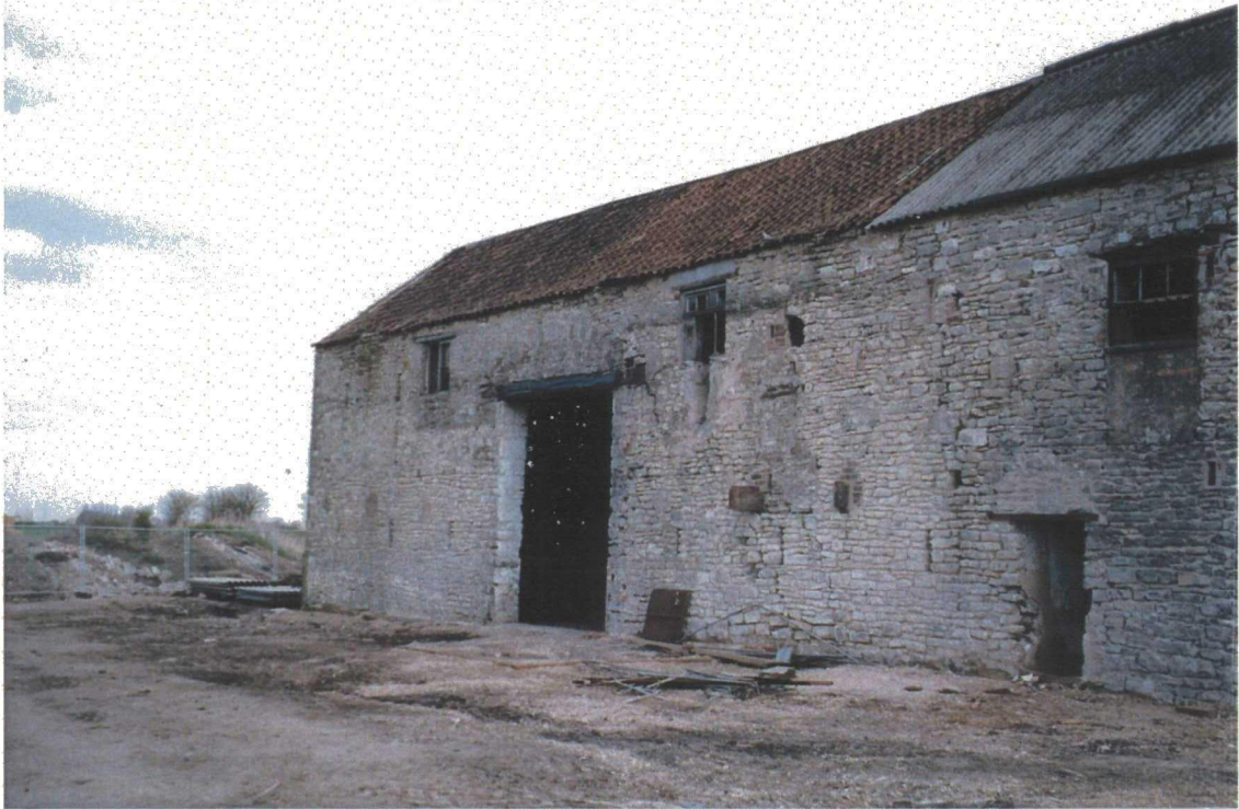
Plate 72. External View of Old Barn after Demolition of Brick and Corrugated Iron Structures
