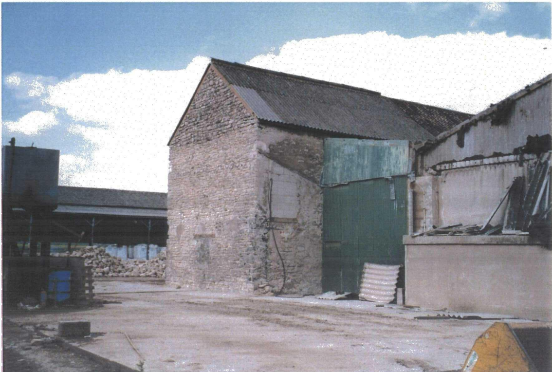
Plate 73. External View of Old Barn after Demolition of Brick and Corrugated Iron Structures
