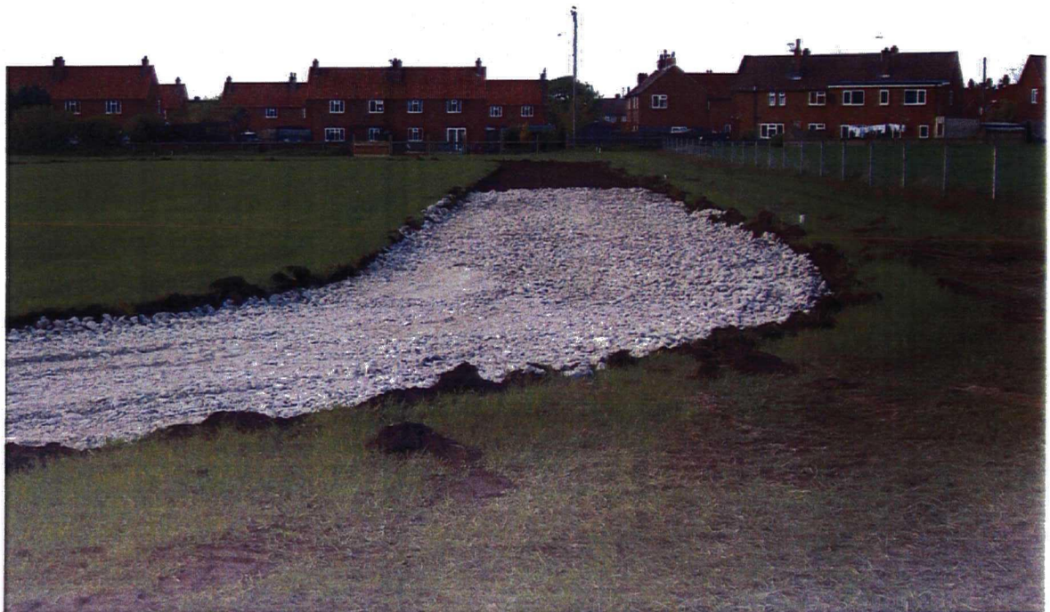
Plate 6. View of Site and Excavated Road and Car Park Area. Facing North West
