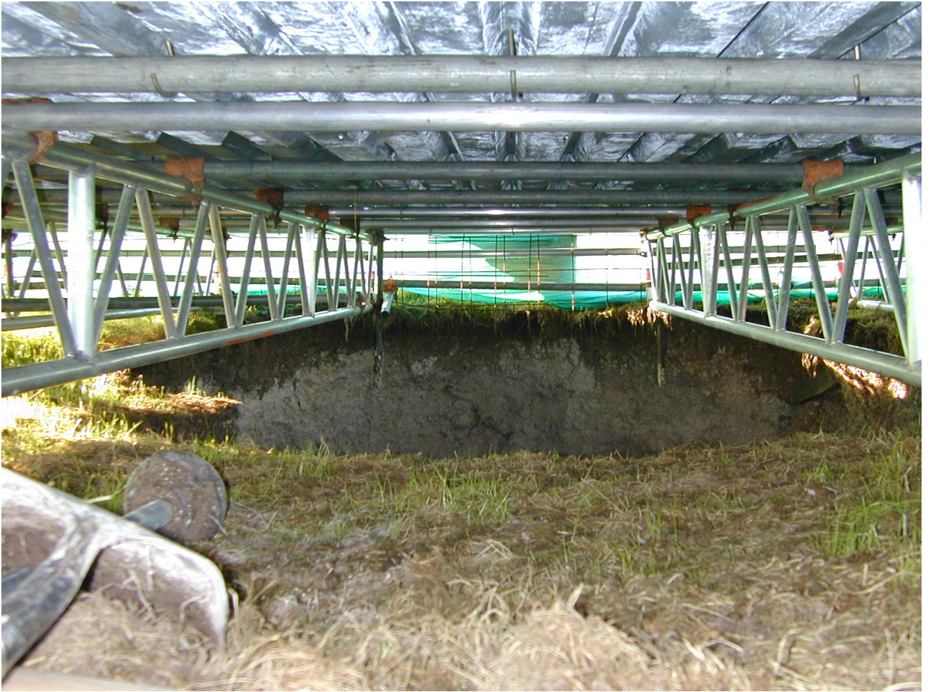
Fig 01 overview of collapse 2
