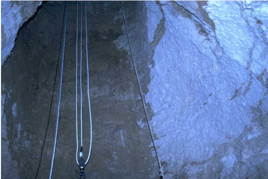
Figure 5: chalk rubble and clay spillage layer in the shaft wall
