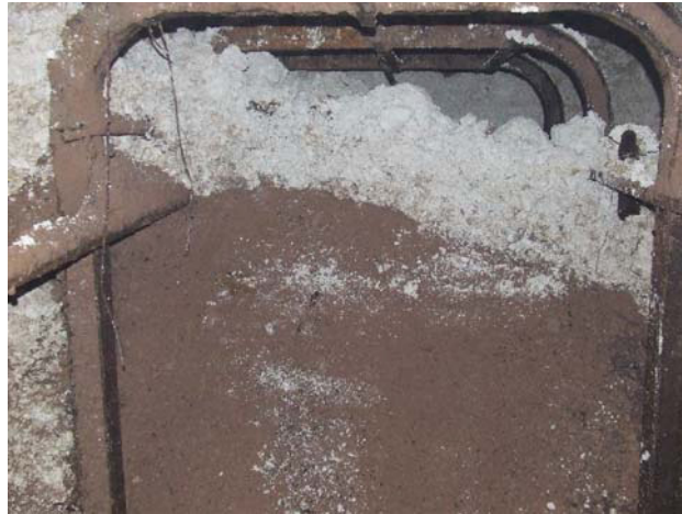
Plate 26: The 1970 road stone used to backfill the tunnel. Compressed by later collapses (photo number 661-6085-01)
