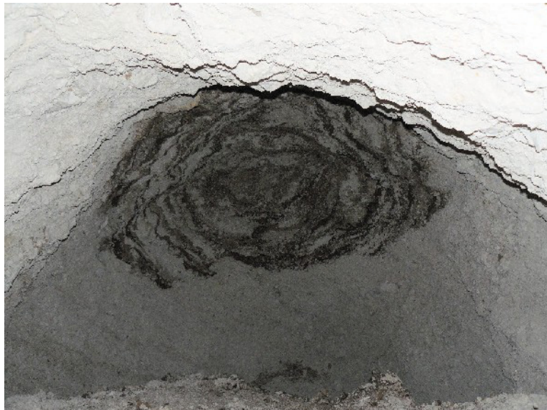
Plate 14: Looking up to the base of organic deposits from the top of a void in the mound (photo Skanska)
