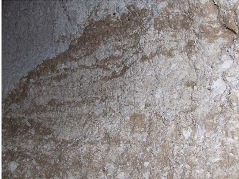
Plate 9: East section of the top of Bank I, as seen in a void above the tunnel (photo number 661-6114-61)
