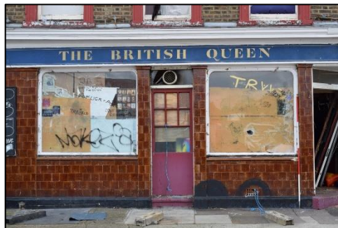
Photo 2: The ground floor windows, glazed tile detailing on the north elevation & the basement chute hatch (below left window)
