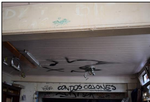
Photo 9: Panelled ceiling and boxed in structural cross beams within the ground floor bar
