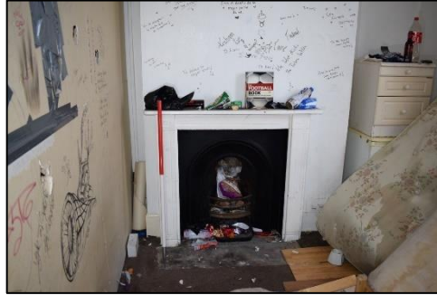
Photo 16: Original 1 st floor mid-19 th century stucco fire surround & cast iron grate
