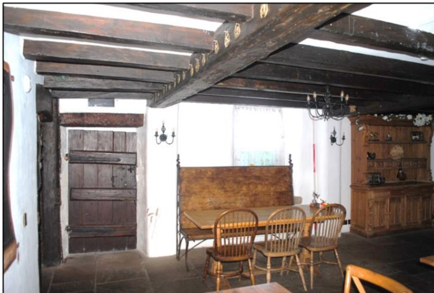
Photo 6. North wall [AB1 – G1] with the front door of Cross Butts on the left
