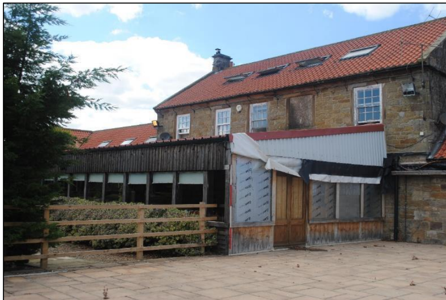
Photo 59. Sun Terrace (S1); poor quality finish to the east gable; view NW
