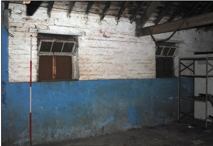
Photo 85. SE corner of the east wall of the Barn; examples of early 20 th century windows
