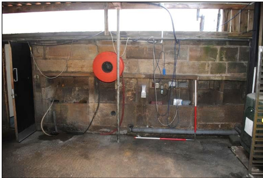
Photo 37. Stone troughs in the east wall of the Kitchen (K1); view west
