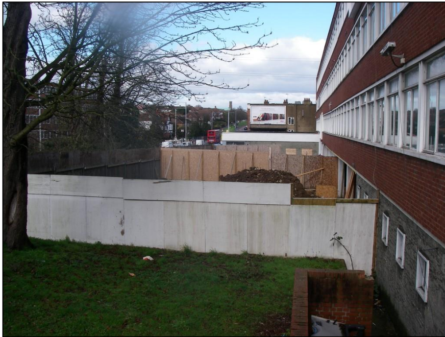
Photo 6: The view towards north-east from the terrace on the south-west facing side of the building, showing the construction works beneath the building extending to the outside
