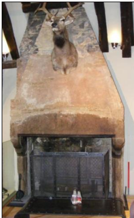
Photo 4: The original Medieval stone fireplace with later brick stack, taken during the site visit
