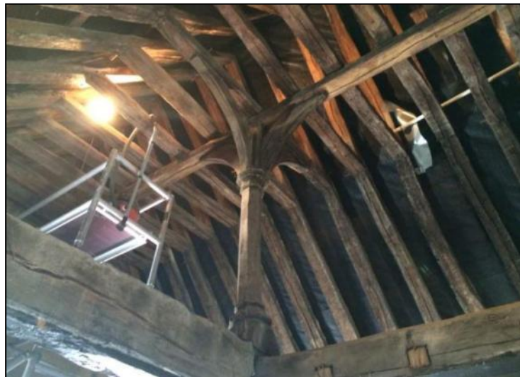
Photo 2: The crown post roof within No. 65 High Street, viewed from the first floor level, taken during the refurbishment works
