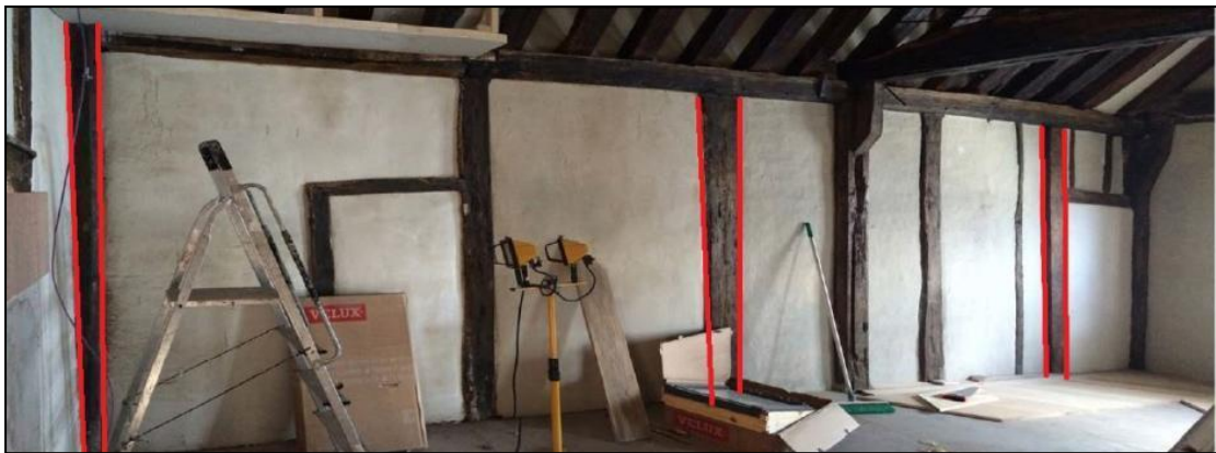
Photo 6: South wall of the 1 st floor. The beams (digitally outlined in red) may mark the previous line of a structure that ran along the position of No. 67 & 69 (taken during conservation works)
