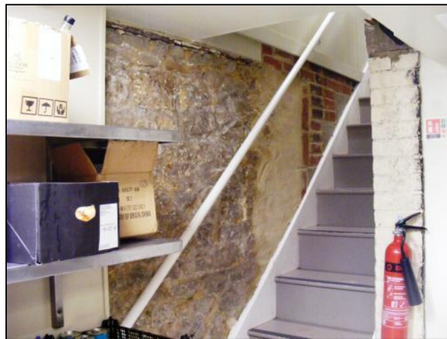
Photo 17: Ragstone wall and sill beam visible in the cellar, taken during the site visit
