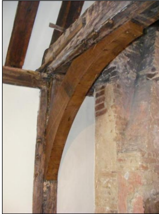
Photo 14: Replacement arch brace on the first floor, taken during the site visit
