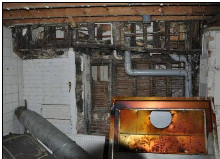
Photo 16: Timber wall studs and blocked window in the south-east corner of the ground floor, taken during the refurbishment works
