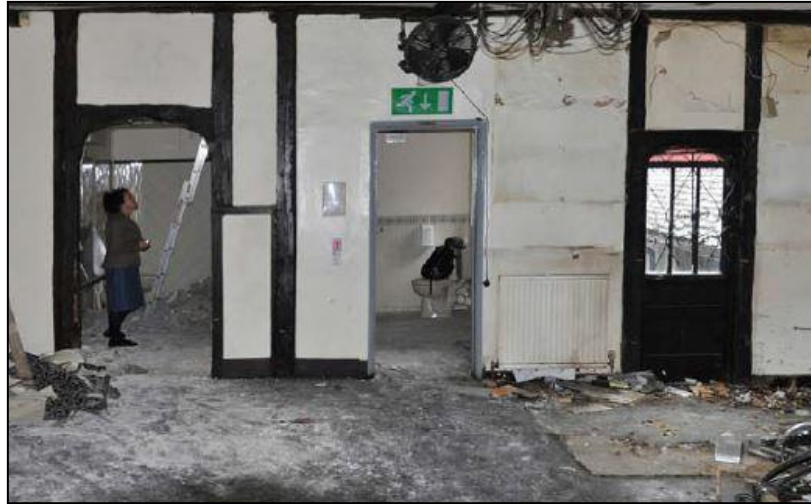
Photo 5: Medieval doorways located on the east wall of the first floor, taken during the conservation works
