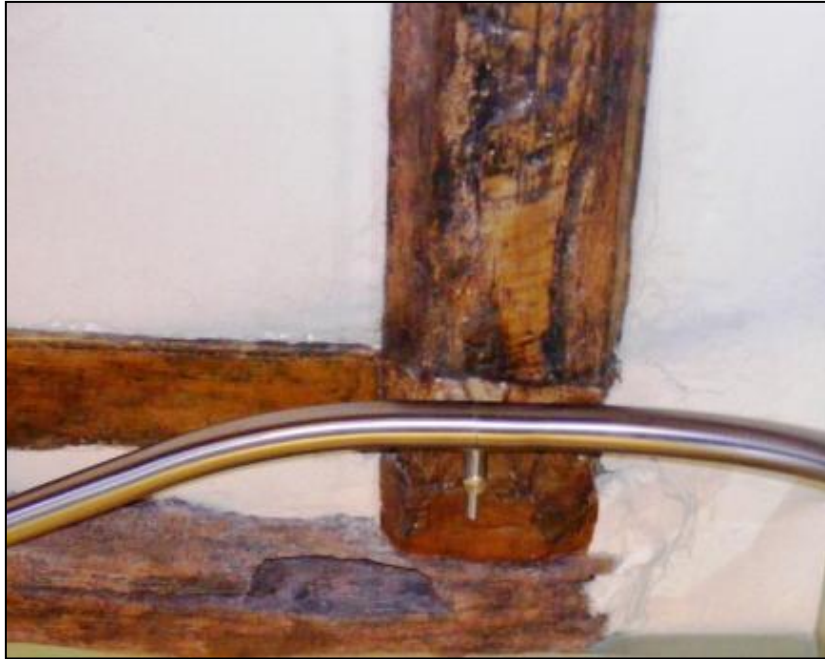
Photo 15: Tooling marks on timber in the stairs area of the building, taken during the site visit
