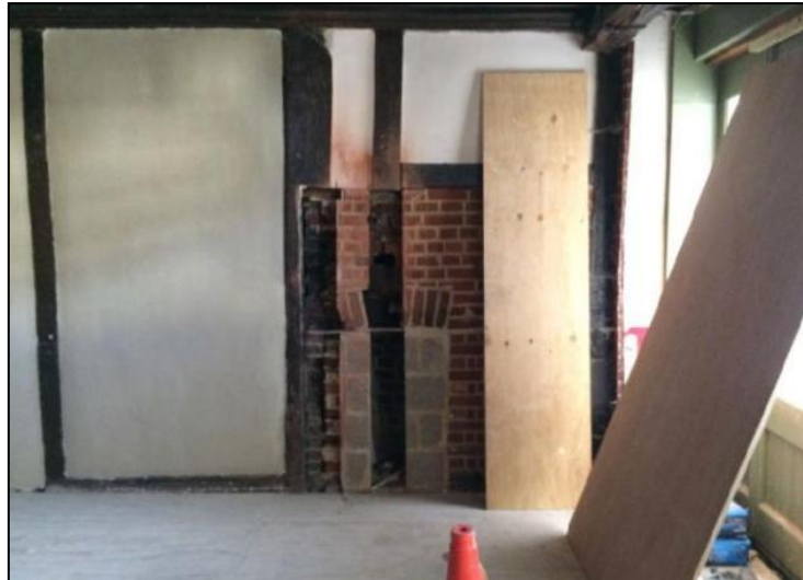
Photo 15: 19 th Century heath and chimney stack located in the south wall of the ground floor, taken during the refurbishment works
