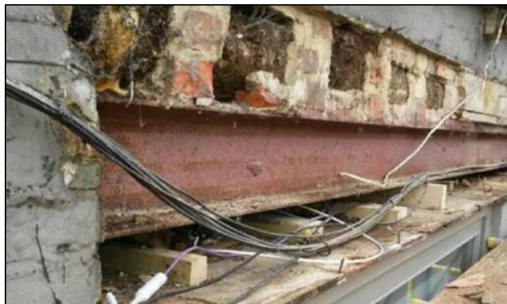
Photo 9: Timber first floor joists located behind the stucco on the front of the building, taken during the refurbishment works
