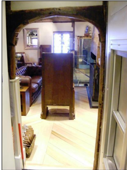
Photo 13: Medieval chamfered doorway on the east wall of the first floor, taken during the site visit
