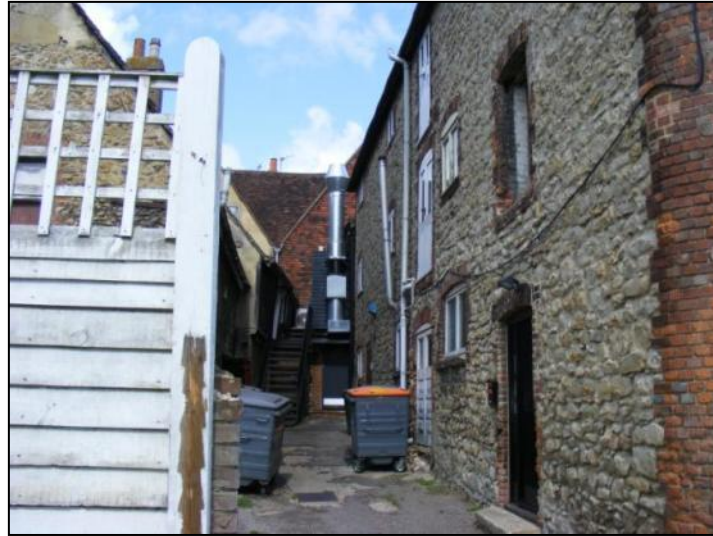
Photo 8: The rear of the properties shows the encroachment of the link block into No. 65 High Street, taken during the site visit
