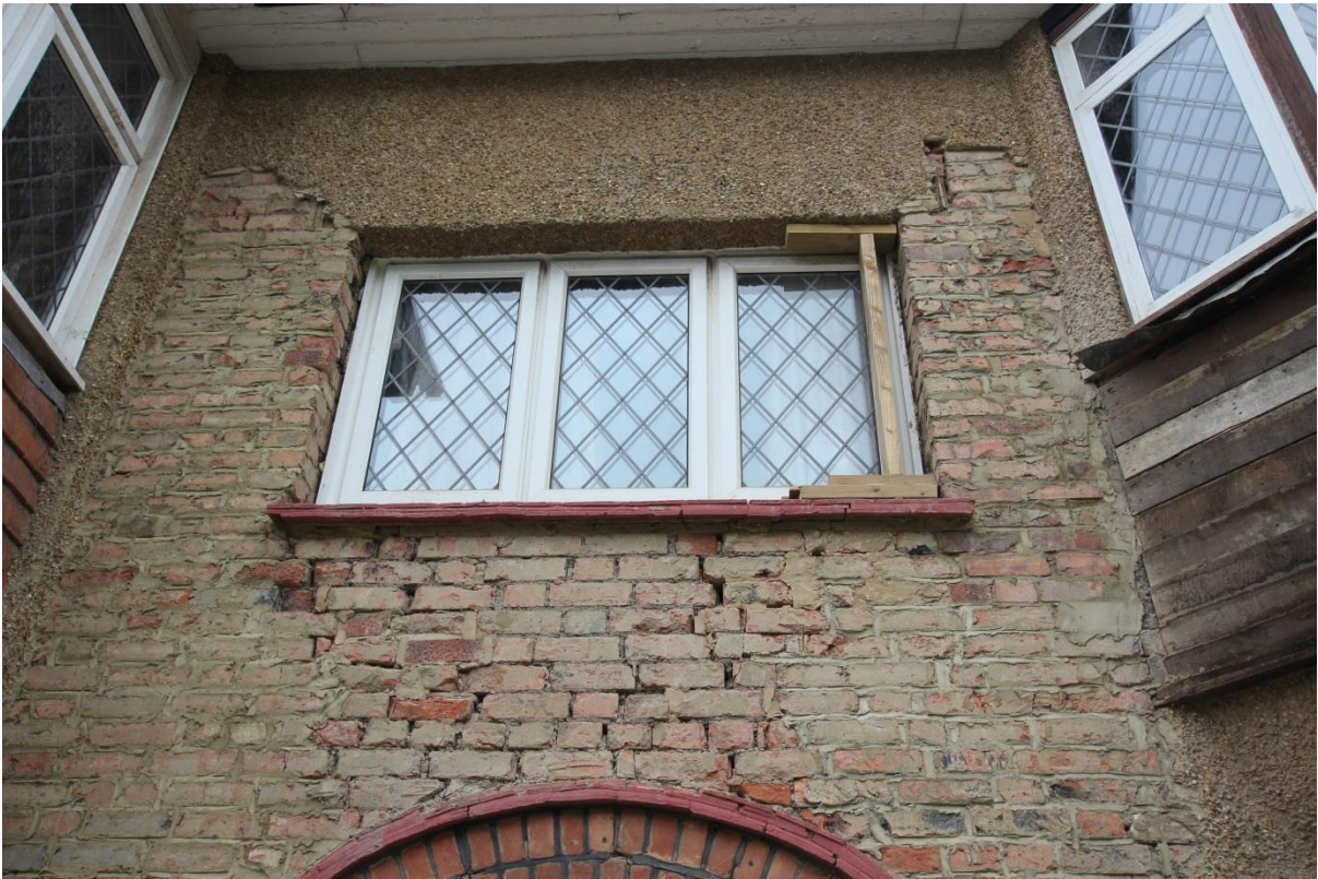
Plate 7: Front elevation first floor window, showing the condition of the brickwork and cracking
