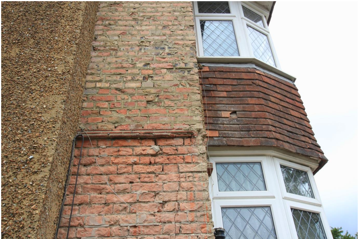
Plate 8: South elevation, adjacent to bay window, showing the condition of the brickwork and cracking
