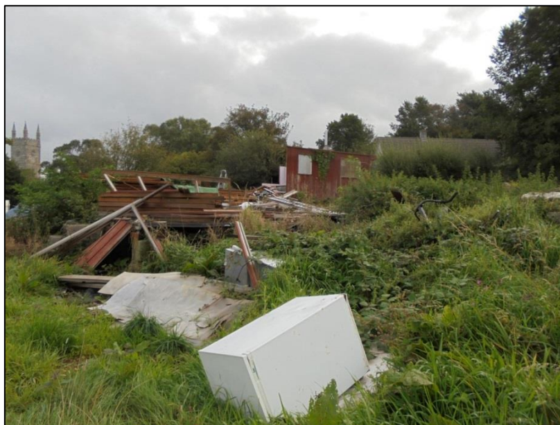
Photo 7: Building debris in field 2, from the south-east of the field looking south-east
