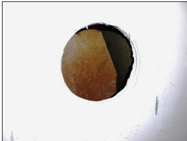
Photo 14: Back of the timber panelling from the waiting room side of the wall
