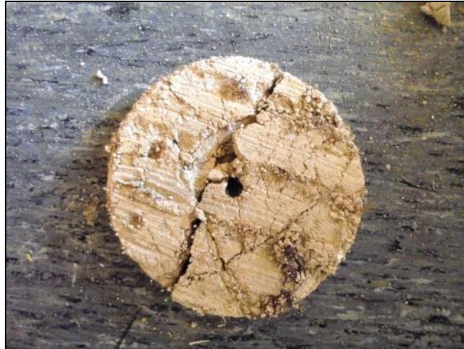
Photo 11: Details of the plaster from the lobby side of the wall, with timber lathe impressions
