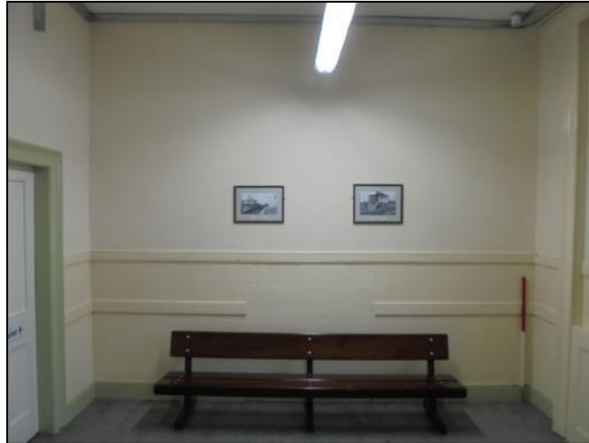
Photo 9: View of the western interior wall of the lobby, from the east, scale 1m
