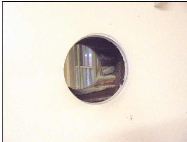
Photo 12: The back of the timber lathes with plaster keying, from the waiting room side of the wall
