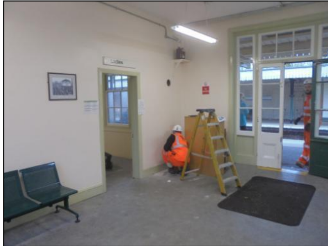
Photo 13: Position of the exploratory holes on the waiting room side of the wall, from the south-east
