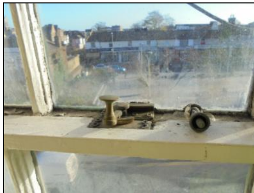
Photo 10: Sash window lever catch, plate and lock on a window in room 8 on the second floor
